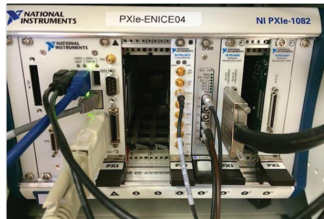
Figure 1: The GMT module installed in slot 5 of a PXI Express crate.
