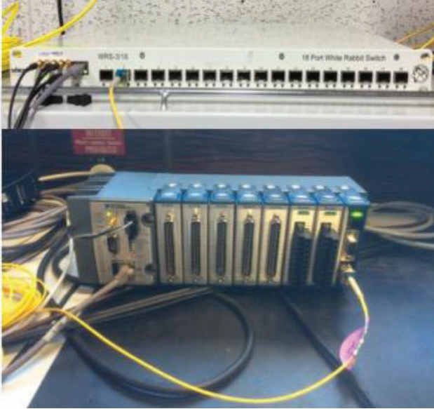
Figure 2: The test setup with the cRIO-WR module connected with the yellow fibre to the WR switch on top.
