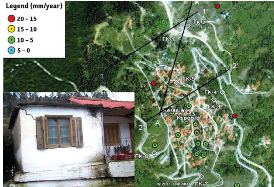
Figure 8. Modelling applications using EO satellite data: measured PSI displacements at Kerasia, Greece. (Moretti et al., 2012). White diamonds represent boring locations. Inset: typical damage.
