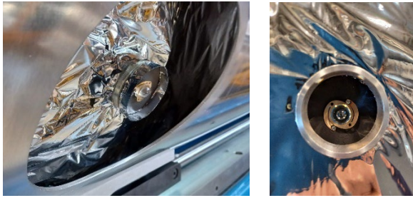
Fig. 8. FSI insulated reflector after installation on the Cold Mass and integration with the Cold Mass MLI.
