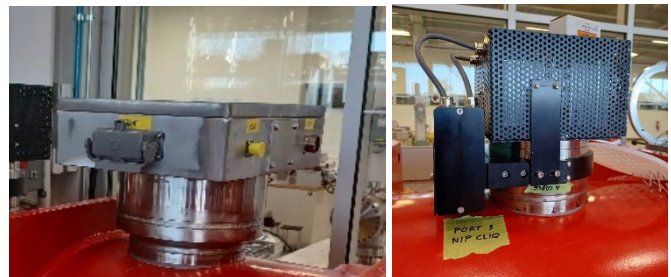
Fig. 19. The warm interface boxes of an IFS (left) and a CLIQ (right).
