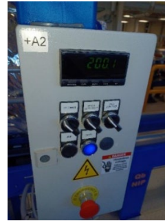
Fig. 11. Local control panel, allowing selection of winches or jacks and providing a readout of winch pulling force or jack elevation.
