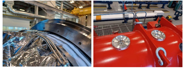
Fig. 10. Capillary tube clearance and warm head position must be visually monitored during cryostating of the Cold Mass assembly.
