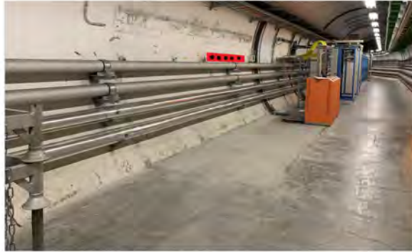
Figure 5 – Proposed location of requested 5 x 220V 16 A power plugs with dedicated local emergency stop (AUL) in UA83.
