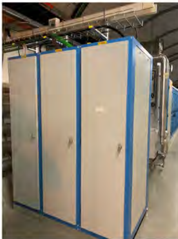
Figure 7 - Rack CYFIB01 in the UA83 gallery.
