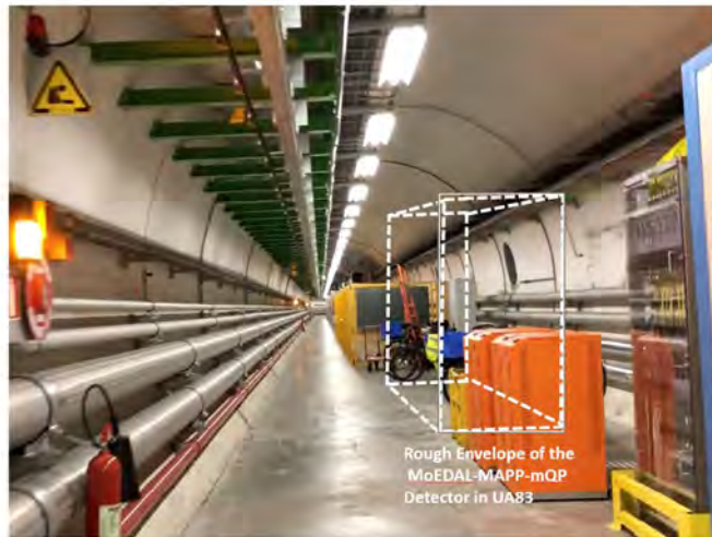
Figure 4 - Indication of rough envelope of the MoEDAL-MAPP-mQP in its proposed location in UA83.
