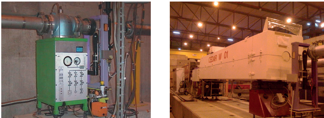
Figure 1.18 – Left image: CET monitor with gas pressure control system. Right image: CEDAR installed in a North Area beam.
