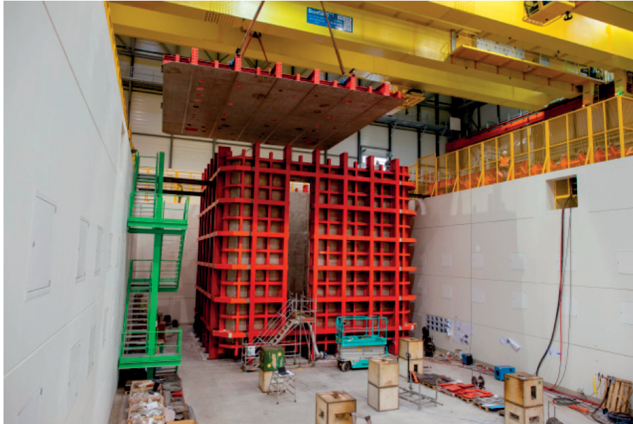
Figure 1.10 – Assembly works carried on the external frame that will host the liquid-argon chamber of NP-04.
