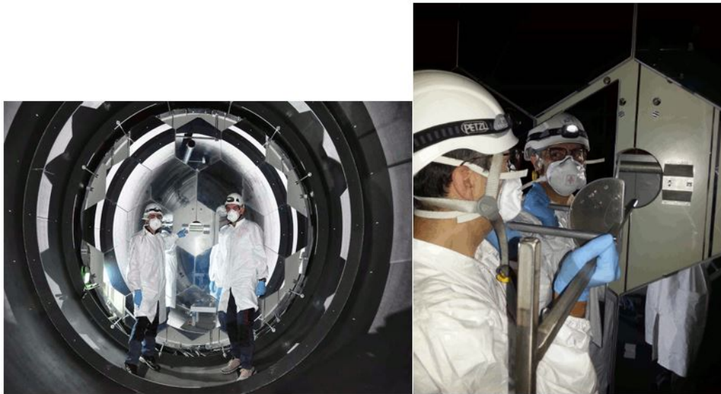
Figure 21: Left: Front view of the mirror system after the two central semi-hexagonal mirrors have been removed. Right: Installation of one of the two new semi-hexagonal mirrors.
