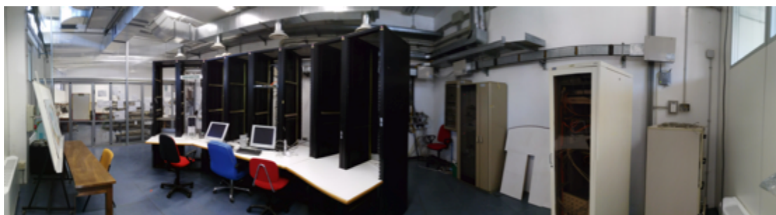
Figure 3.21: New BTF control room.
