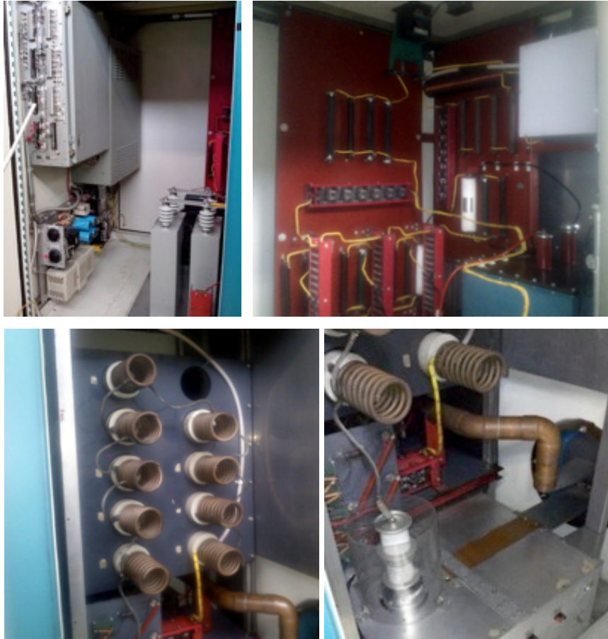
Figure 3.3: The SCR rectifier, the core bias and filament power supplies are placed inside one door of the modulator racks (top left), together with the diode arrays, the large charge capacitor and filters of the charging circuit (top right). In the other rack door: the 9 LC cells PFN (bottom left), the Hydrogen gas thyatron and the conductor towards the pulse transformer (bottom right).
