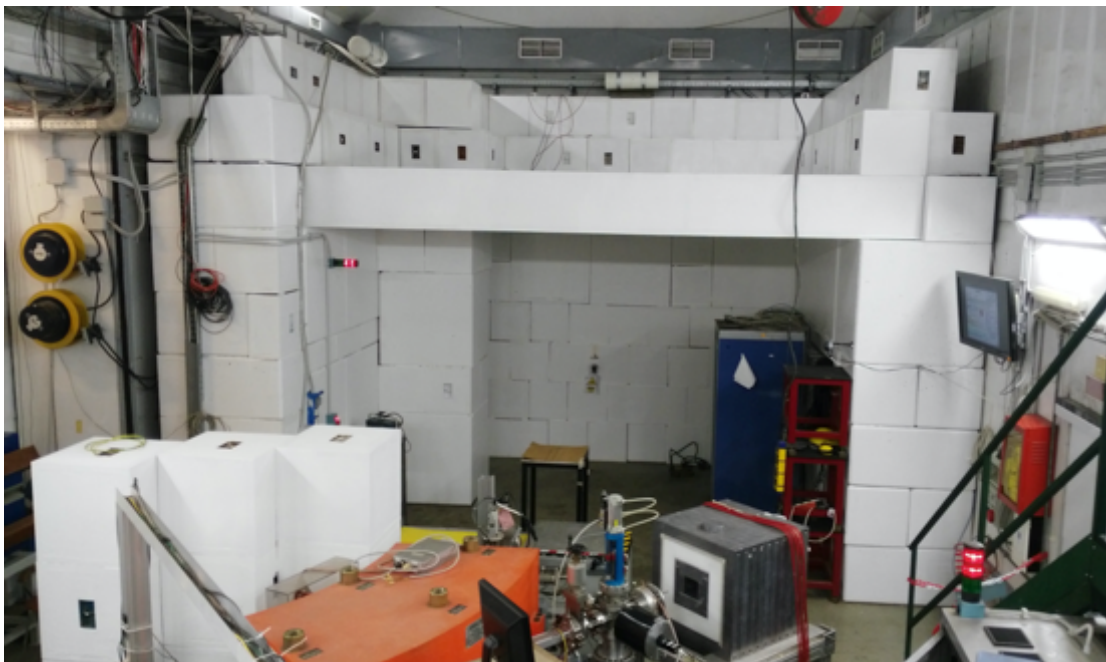
Figure 2.10: During the July-September 2015 shutdown the concrete block shielding of the BTF experimental hall has been dismantled and reinstalled in an improved configuration, adding a concrete ceiling (50 cm concrete).
