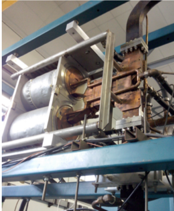
Figure 3.6: The SLED device is composed by two (cylindrical) resonant cavities, connected by a 3 dB hybrid coupler, taking as input the power from the klystron (just below, not shown in the picture) and output to the waveguide network towards the accelerating sections.
