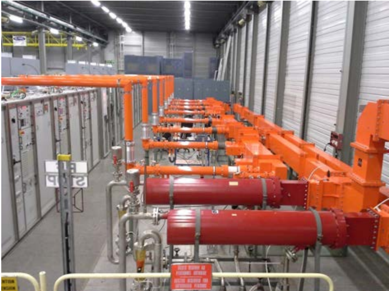
Figure 23: The new, IOT based 800 MHz power plant for SPS in BB3
