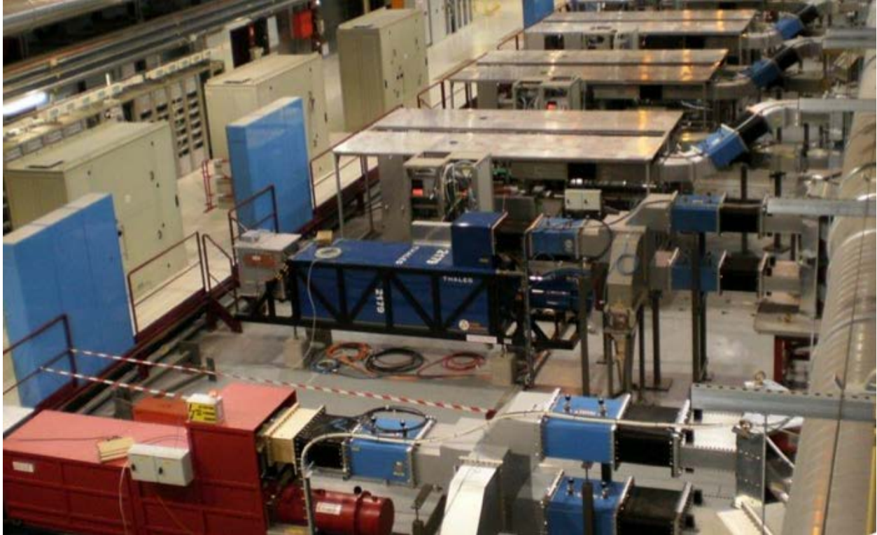
Figure 36: View in the Linac4 equipment room in 2014
