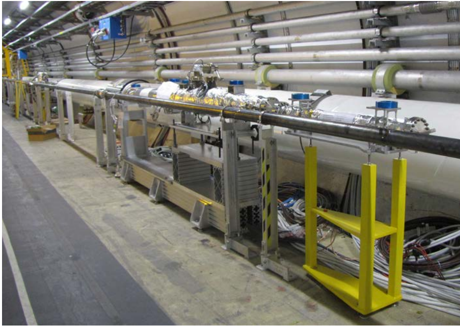
Figure 9: The prototype beam gas vertex detector vacuum system installed in LSS4 of the LHC.
