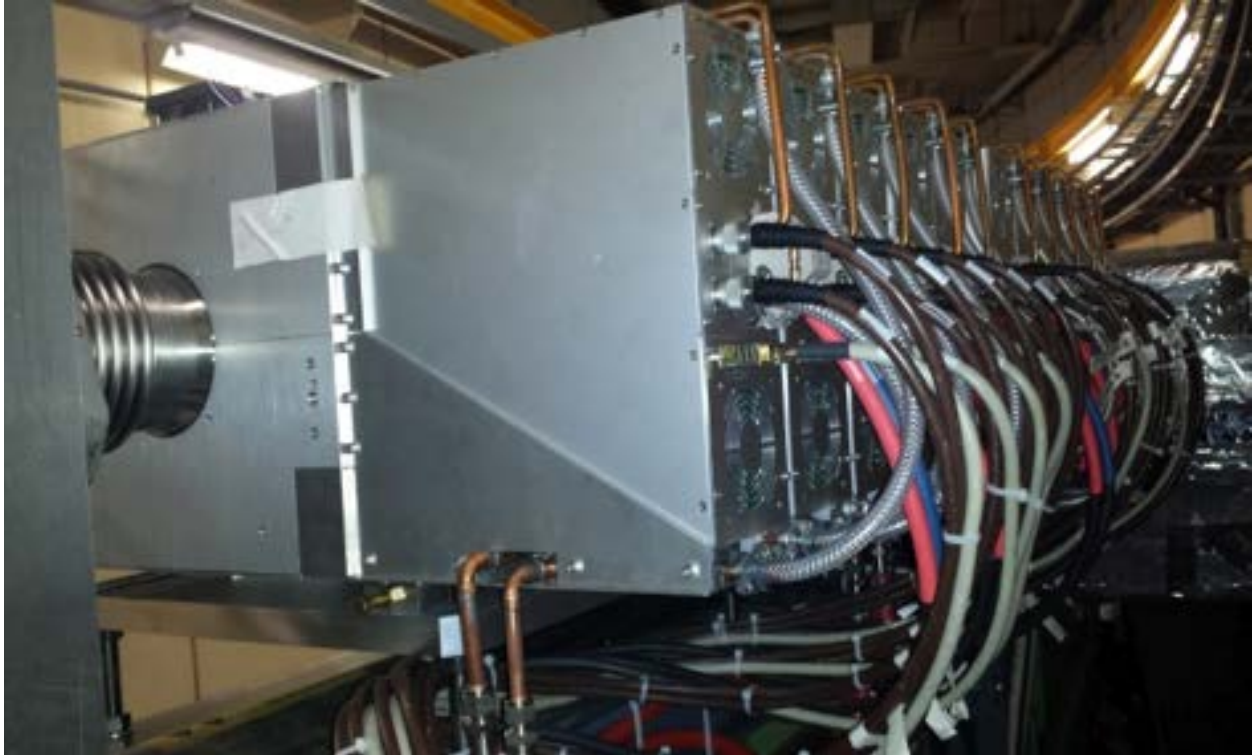
Figure 26: Ten-cell prototype Finemet® cavity system installed in PSB ring 4.
