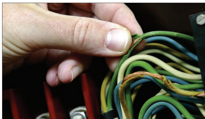
Aging and ionizing radiation degrades the insulation on the PS dipoles' pole-face winding. This is one reason for the renovation.
