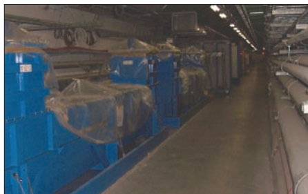
One of the PFN modules installed in the LHC.
