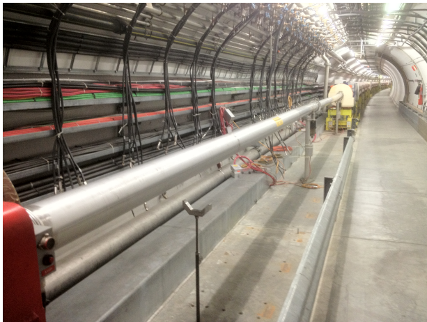
FIG. 2. Precise location in LSS3 of the SPS where the new kicker system will be installed. About 13 m of longitudinal space is available, but only about 8 m of that space is usable because of beam aperture (stay-clear) considerations.
