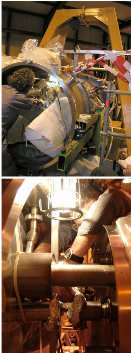
Figure 6-12: Pictures of the intervention inside the Cryostat. Top: Welder working on the MFB side. Bottom: welder working on the MRB side.
