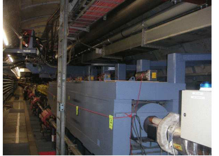
Fig. 8. Installation of beam loss detectors on top of the HERA proton beam dump.
