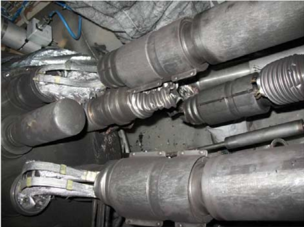
Figure 15: Damage to interconnection QBQI.27R3 by excess extension
