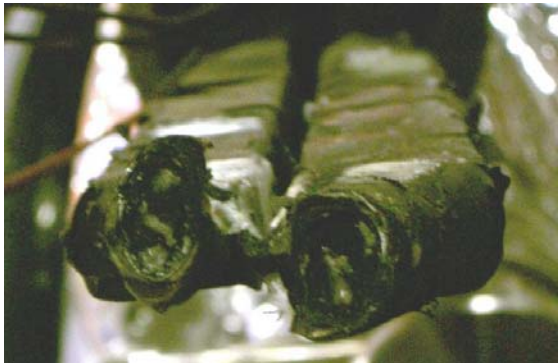
Figure K2: RQD bus-bar following the String 2 incident
