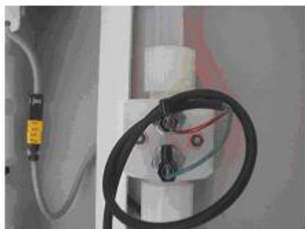
EP U/I test cell integrated into the EP acid line towards the cavity
