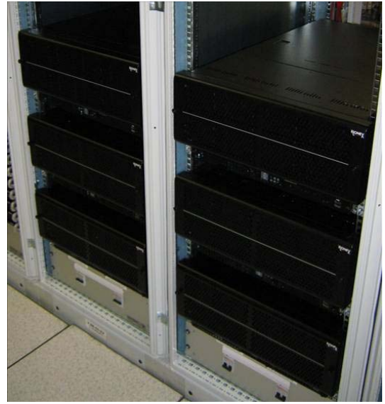
Fig. 1. The six final SFO machines, mounted in two racks.
