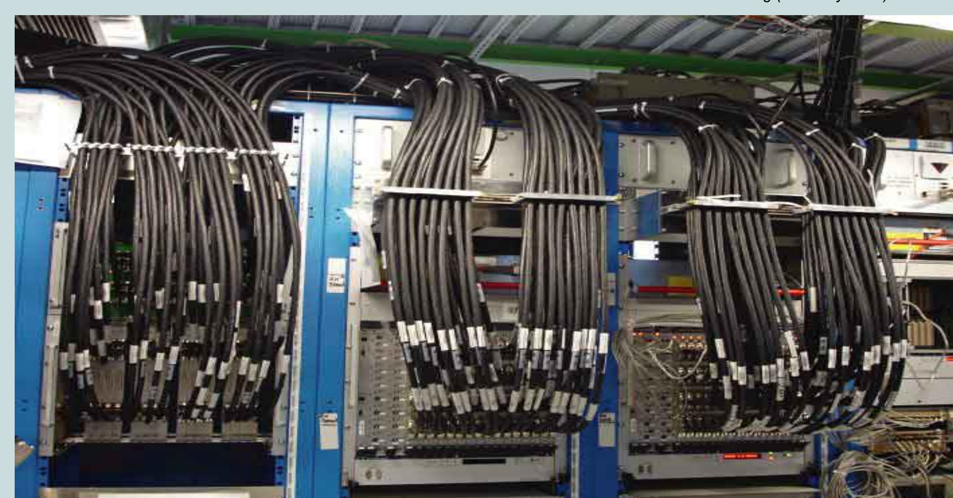
Analogue trigger cables installed in the ATLAS counting rooms. Almost all 776 cables are installed and tested, the analogue receivers and patch panels are also in place.
