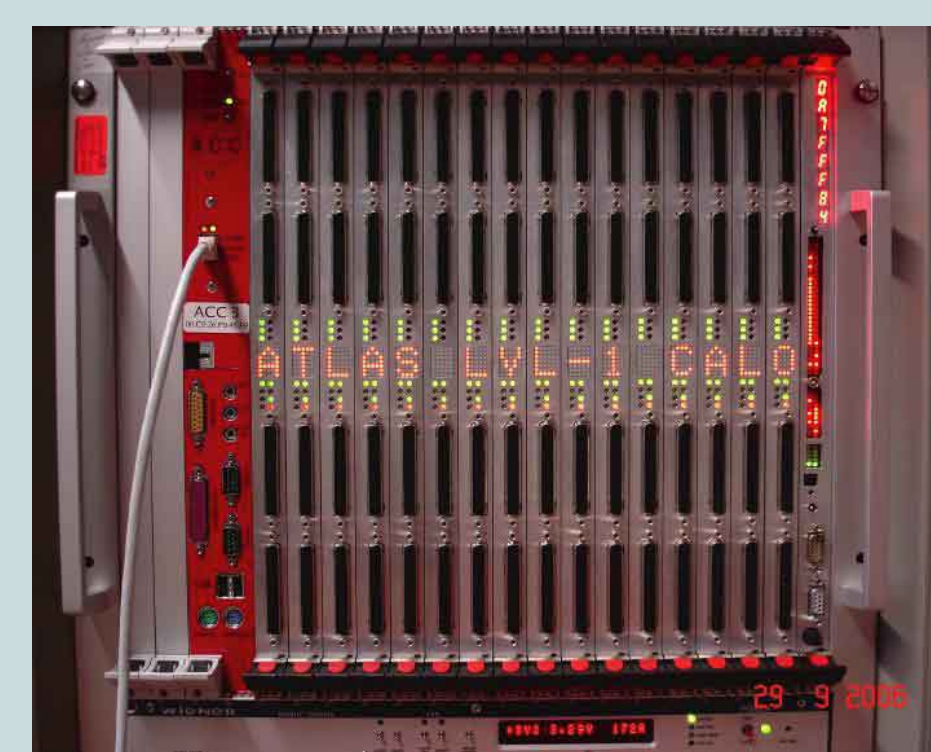
A full crate of pre-production PreProcessor modules of the LVL1 calorimeter trigger. Most of the functionality of these modules is on replaceable Multi-Chip Modules (MCMs). These MCMs each contain a processing ASIC and four ADCs. All the MCMs (3000) are available and final production of the 124 PreProcessor modules is in full swing (February 2007).
