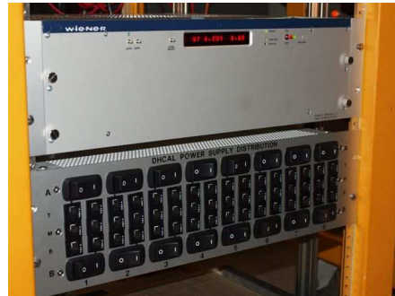
Figure 4: Photograph of the Wiener low voltage power supply and the distribution box.
