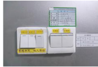
reminder on the switch
