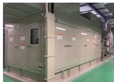
On-site cogeneration system
