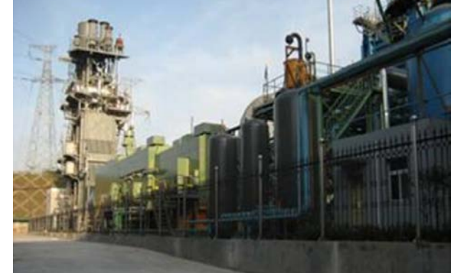
Hydrogen Co-firing Gas Turbine
