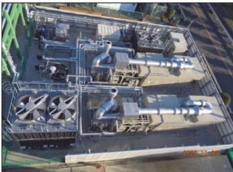
Figure 6 Panoramic view of completed facility
