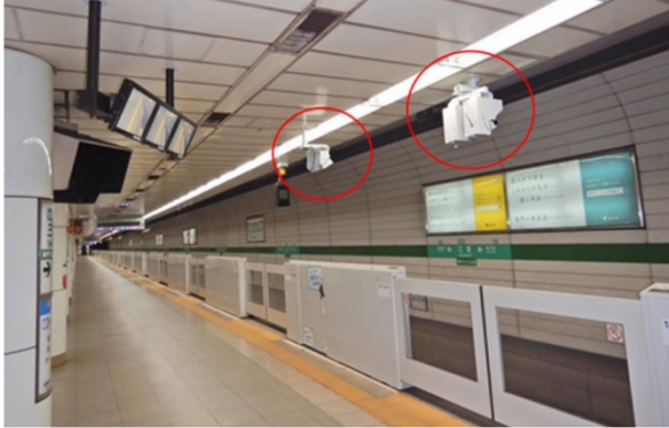
Figure 4 Installation of sensors for interlocking control relying solely on platform-installed equipment at Sannomiya Station
