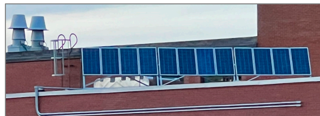
Figure 8. PV panels setup at the rooftop of the MUN core science building.
