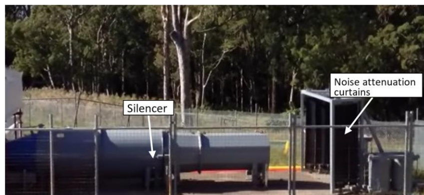
Figure 3. Stage 0 silencer and noise attenuation curtains at the end of the detonation tube.
