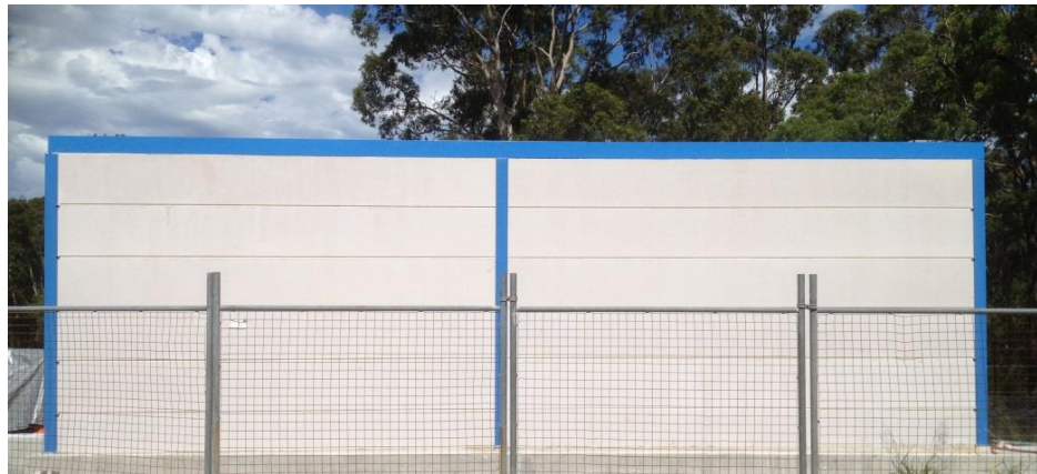
Figure 6. Stage 2 autoclaved aerated concrete-based enclosure outside the bottom ash enclosure.
