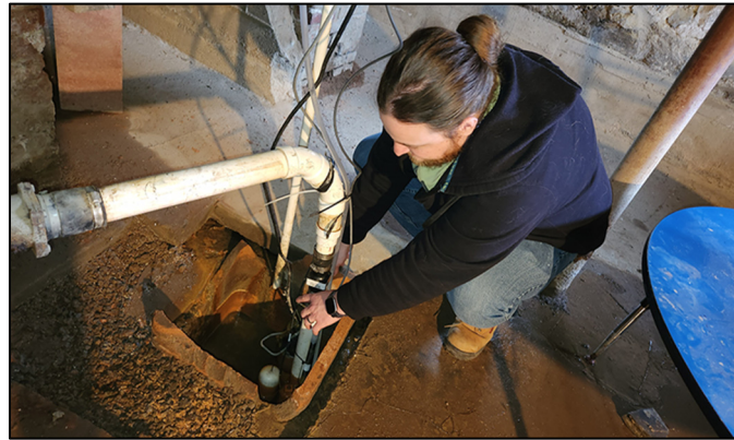
Figure 4. Installation of an MX2001-04-TI-S OnSet© water level sensor and a pHionics© STs series conductivity/salinity sensor located along the side of a drain pipe within a sump pump pit in the Jones house basement.
