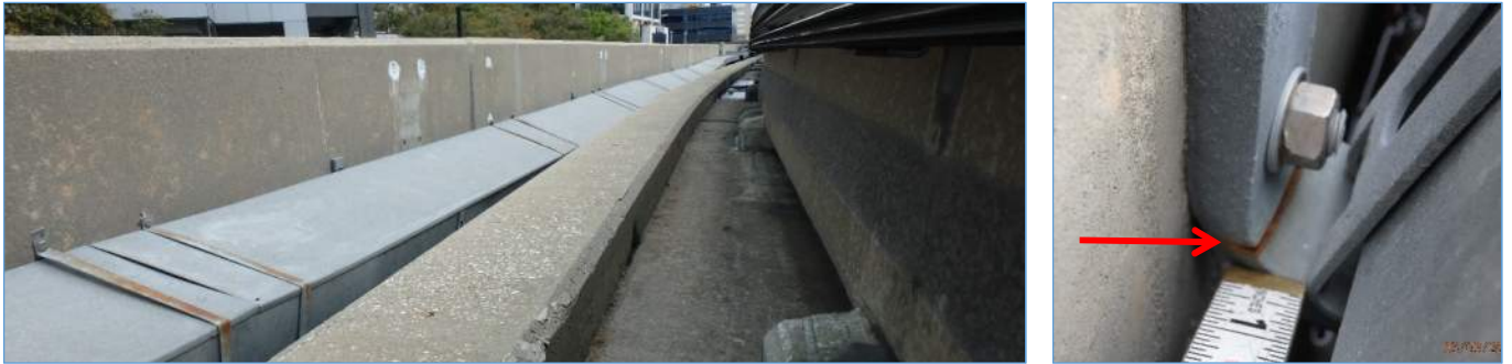
Span 43N Cable Tray with Four Broken Attachment Brackets
