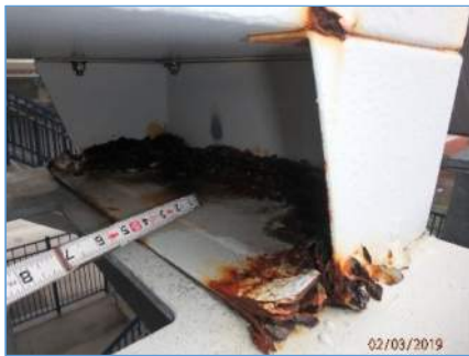
Heavy Corrosion on Electrical Cabinet Legs in Span 409R
