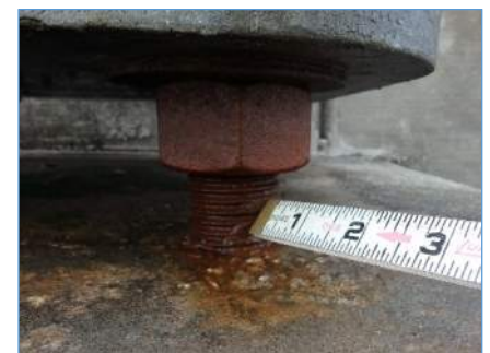
Surface Corrosion on Traffic Signal Pole Anchor Bolts in Span M2
