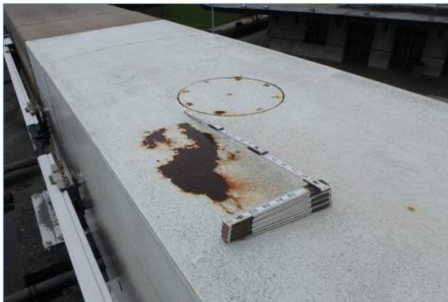
Span 8S: Surface Corrosion on Steel Guidebeam
