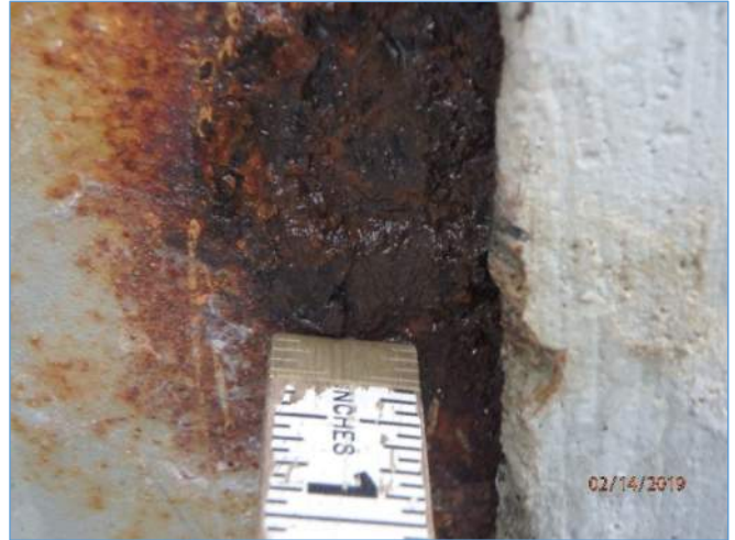
Span 236L: Closeup of Corrosion and Section Loss
