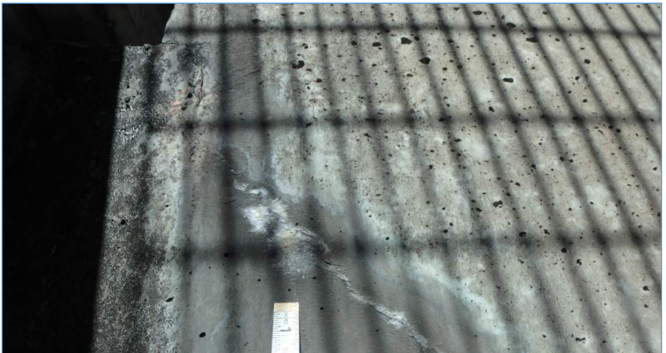
Pier 62: Diagonal Crack Extending Downward From the Left Beam Seat Corner
