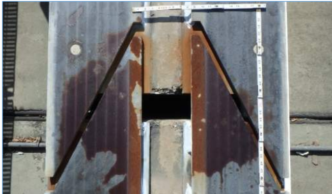
Pier 250L: Surface corrosion on the sliding plates
