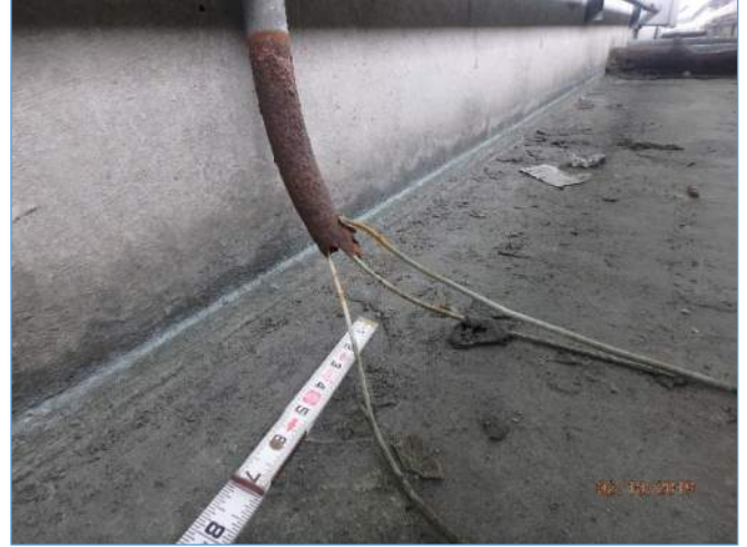
Span 238L: Conduit with 100% Loss Exposing Wires
