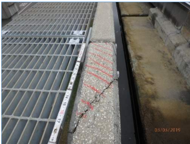
Span 19S: Delamination, Top of Left Sidewall
