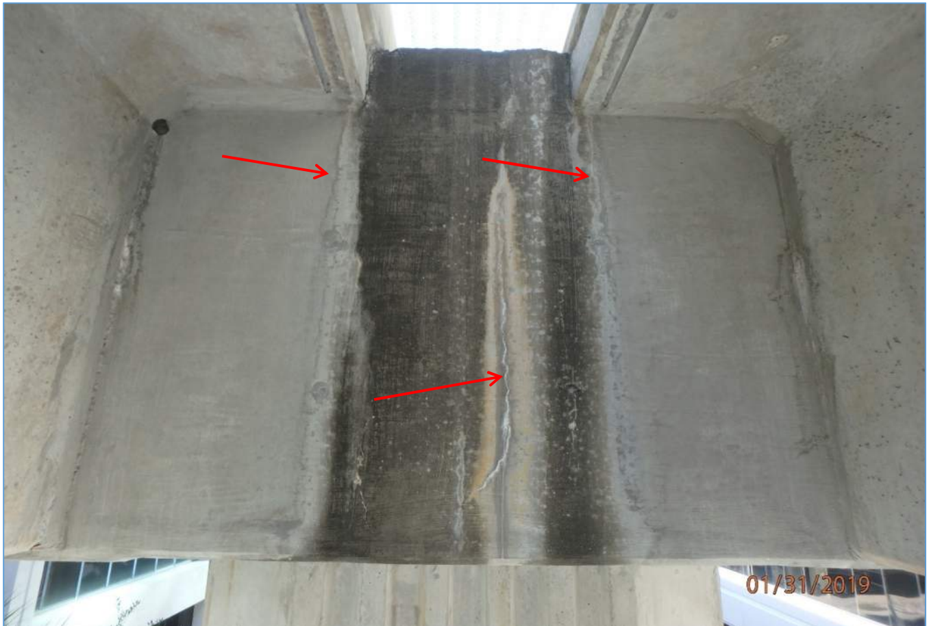
Typical Negative Moment Crack, Full Depth of Cap, Rear Face of Pier 208
