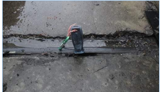
Pier 205R: Typical Seal Adhesion Failure
