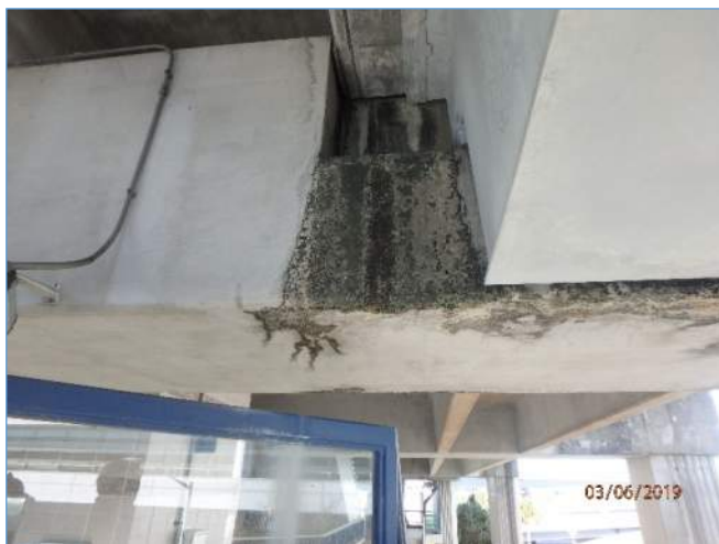
Pier 237R: Staining on Pier Cap
