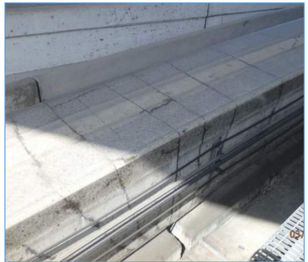
Span 253: Vertical/Transverse Cracking in Guidebeam
