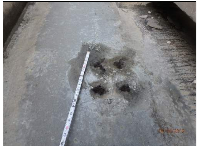
Span 231R: Lift Point Patch Failure
