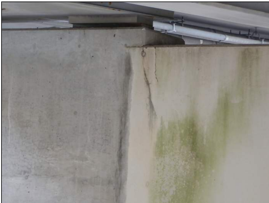
PHOTO 20 – ELEMENT 234 VIEW OF THE CRACKS IN THE SOUTH FACE OF PIER 1, ADJACENT TO THE PEOPLE MOVER PORTION OF THE PIER
