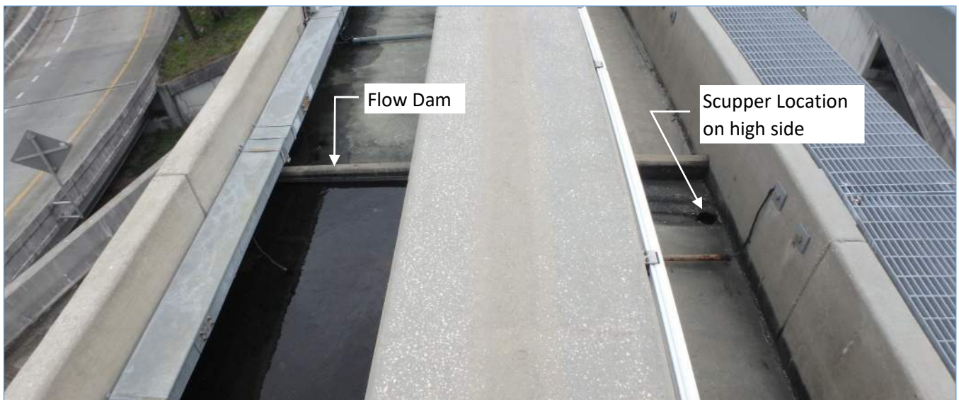
Pier 242R: Guideway, Looking Back Showing Standing Water on the Low Side and Scupper on High Side
