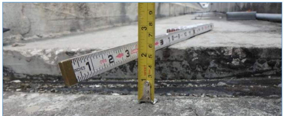
Pier 258L: 1-1/4" Elevation Difference Between Top of Deck and Top of Pier
