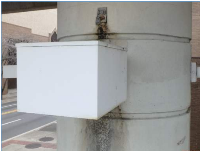
Pier 76: Overview of Water Leakage from Electrical Components
