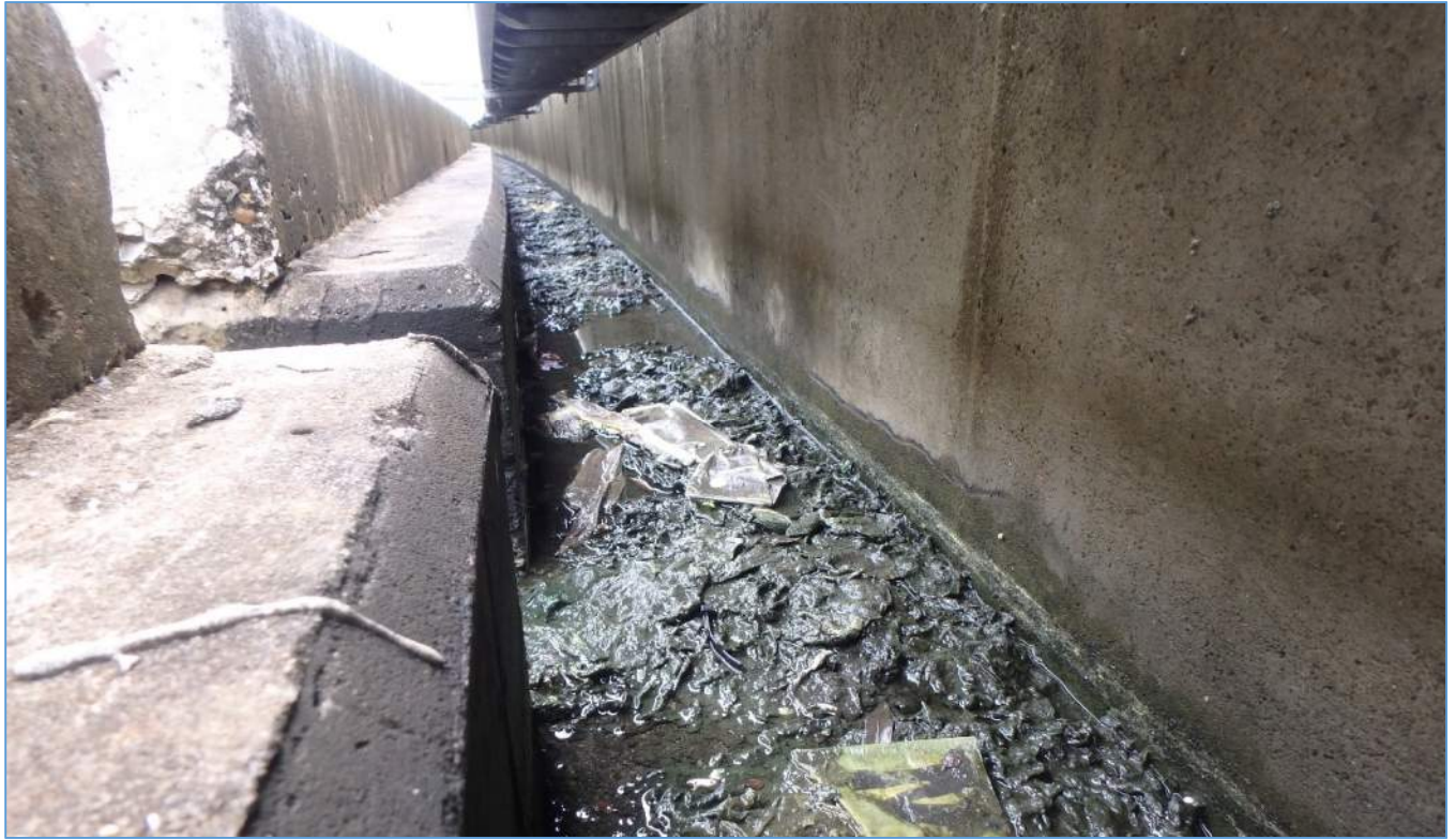
Span 20S: Wet Debris Accumulation, Right Side of Second Pour
