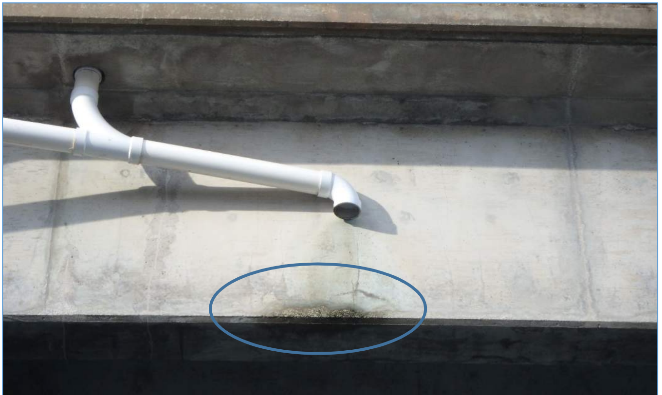
Span 42S Cross: Drain in Need of a Downspout
