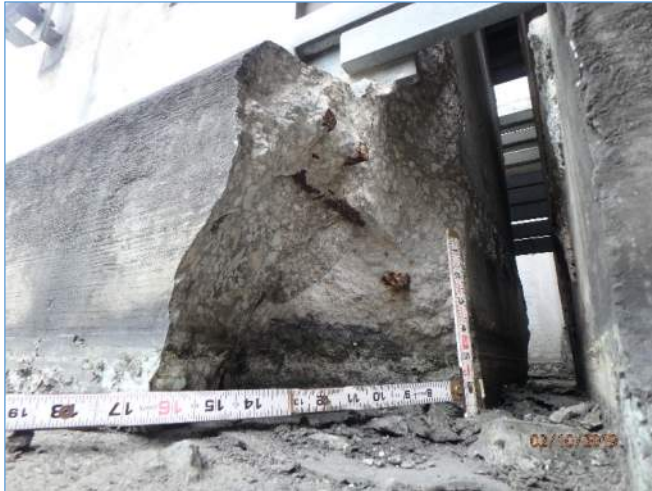
Pier 237: Large Pedestal Spall at an Expansion Joint
