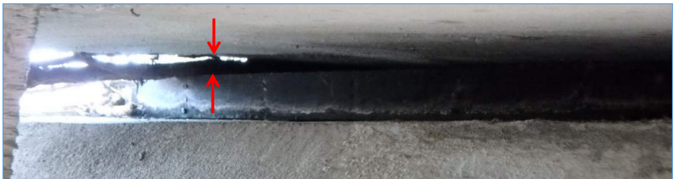
Span M2: Up to 1" Gap for 15" Between Beam and Bearing Pad at Pier M3
