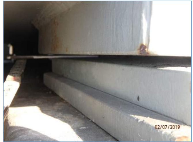
Span 257R at Pier 258R: 1/4" Gap; no right bearing
