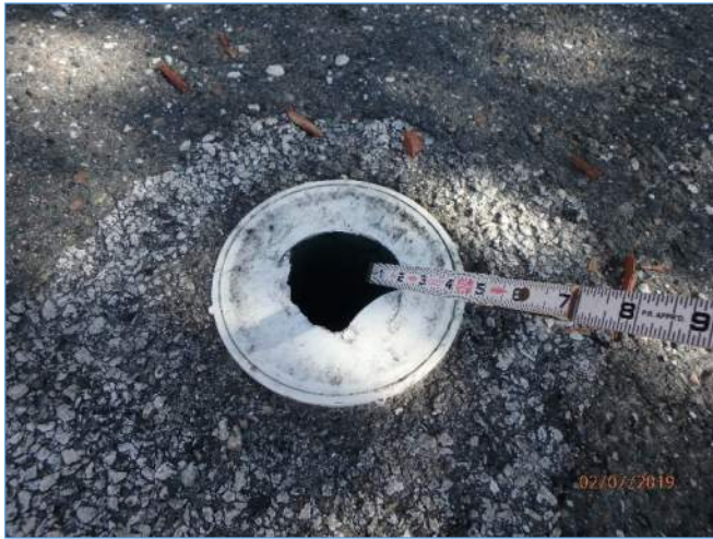
Pier 261R: Broken Riser Pipe Cap
