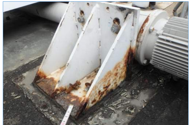
Span 233L: Section Loss on Bolts and Motor Bracket
