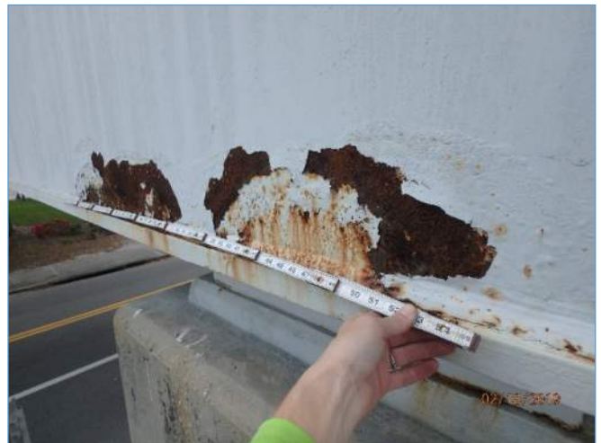
Pier 10N: Corrosion on Cross Girder
