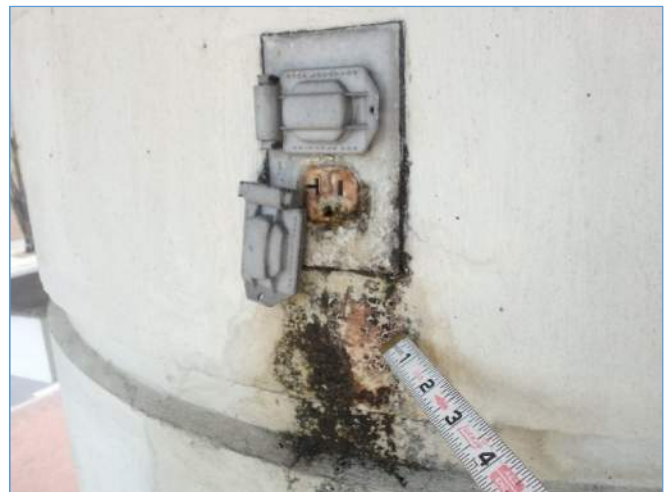
Pier 76: Close-up of Water Leakage from Electrical Outlet
