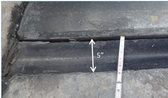
Pier 232R: Joint Width Exceeds Seal Capacity
