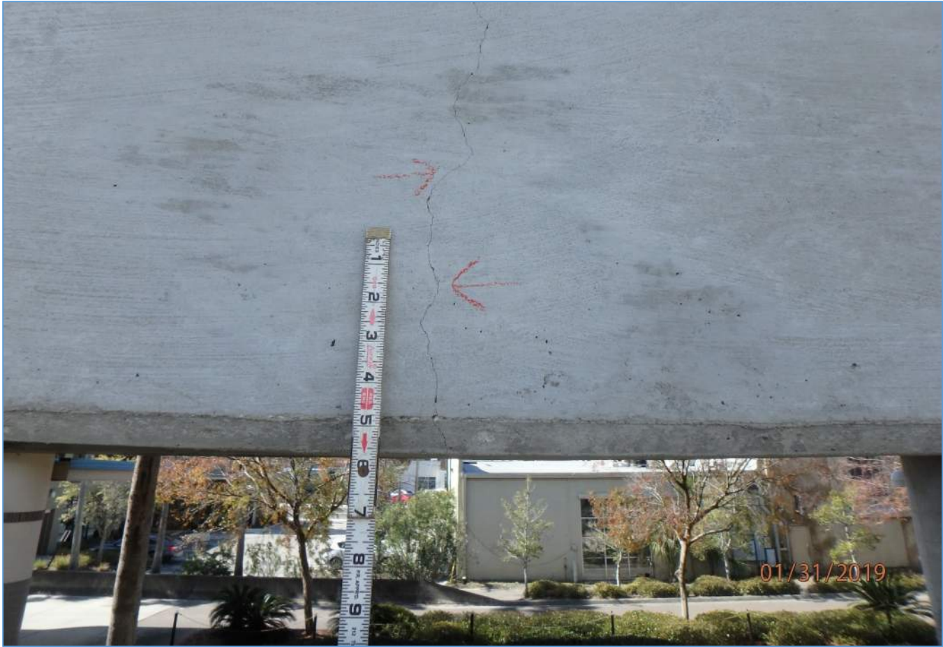
Span 203R – Typical Unsealed Flexural Crack in Cast-In-Place Beam Stems
