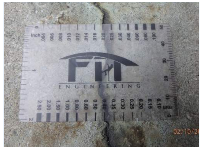
Span 241R: Closeup of Transverse Deck Crack
