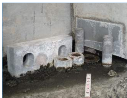
Keeper Plate not Installed
