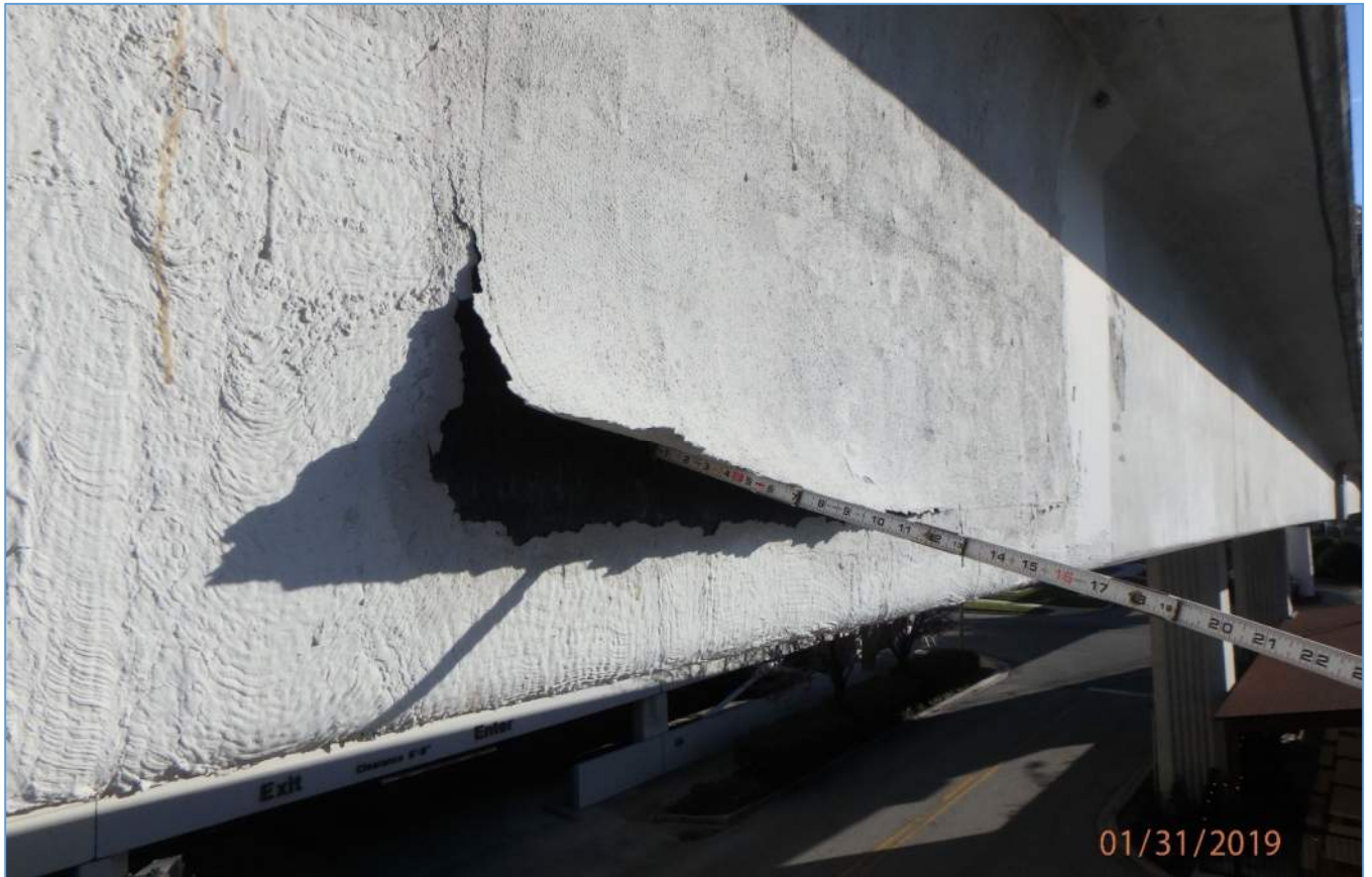
Span 227L: CFRP Failure in at Pier 228
