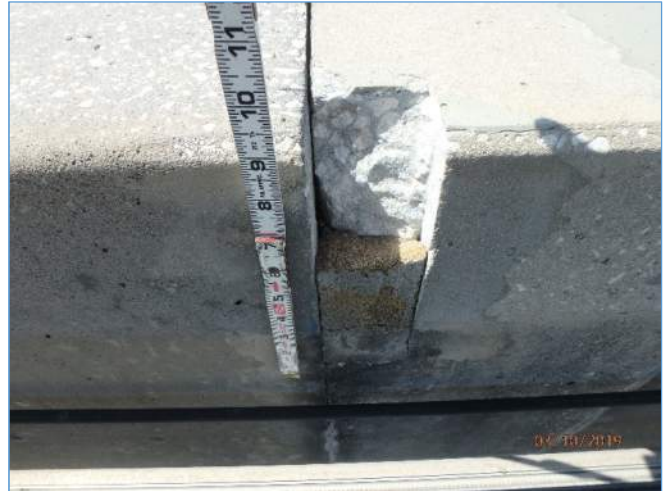
Span R-2L: Failed Patch on Left Side of Guidebeam
