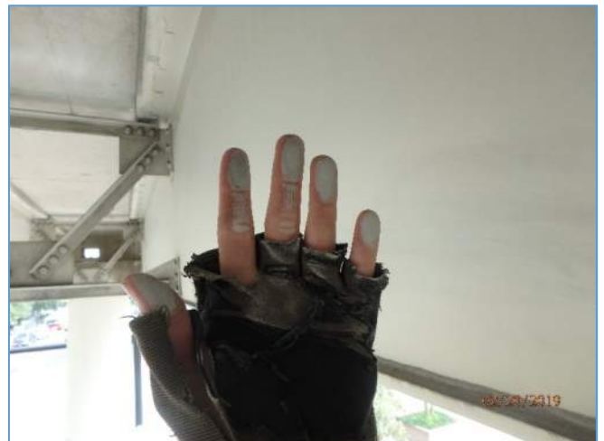
Very Chalky Paint Exterior – Typical Throughout
