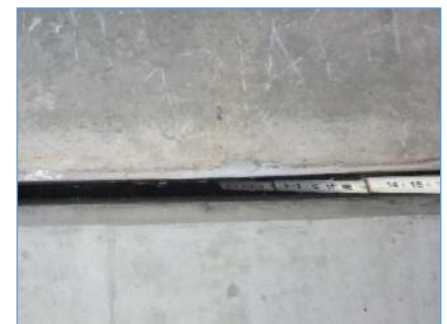
Missing Pad at Pier 62R
