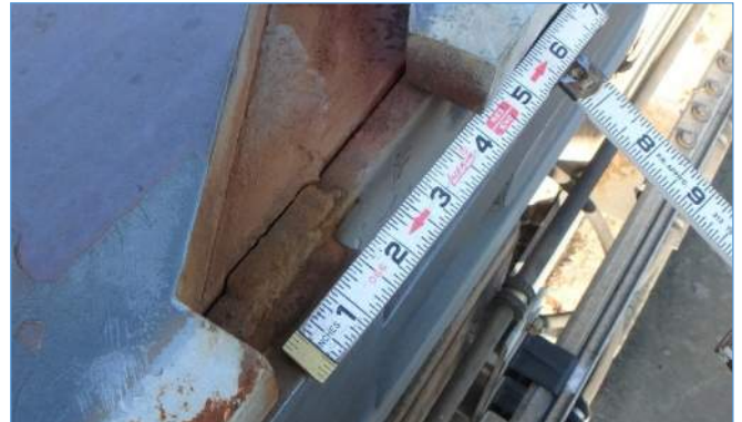
Pier R-1: Tack Weld Crack
