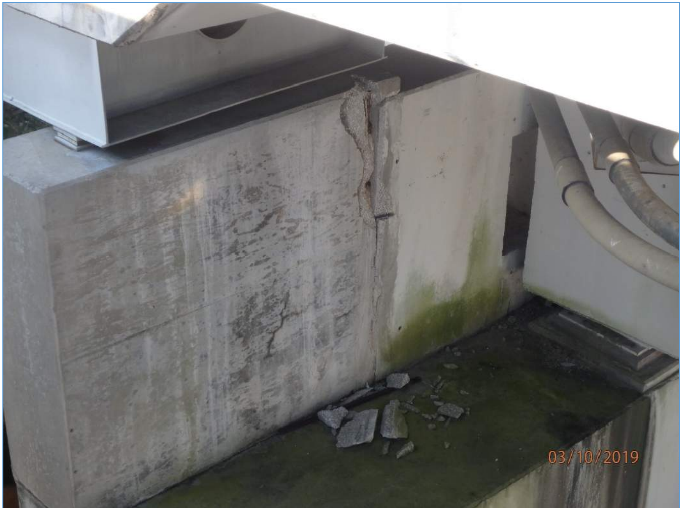
Acosta Bridge Pier R1 LT: Overview of Pedestal Spalling on Front Face
