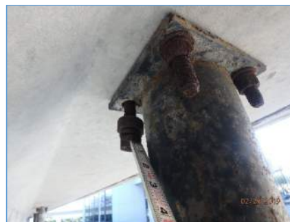
Heavy Corrosion and Bent Bolt for the Traffic Light in Span 55L
