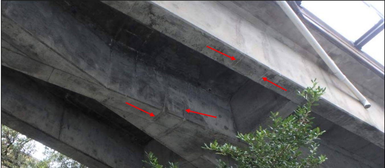
Span 42S – Cross: Typical Sealed Flexural Cracking in Beam Stems
