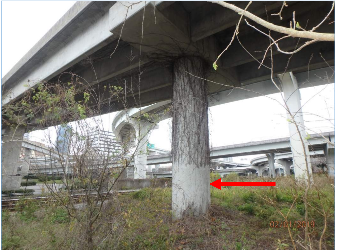
Pier 403: Cut Vines Growing on the Column
