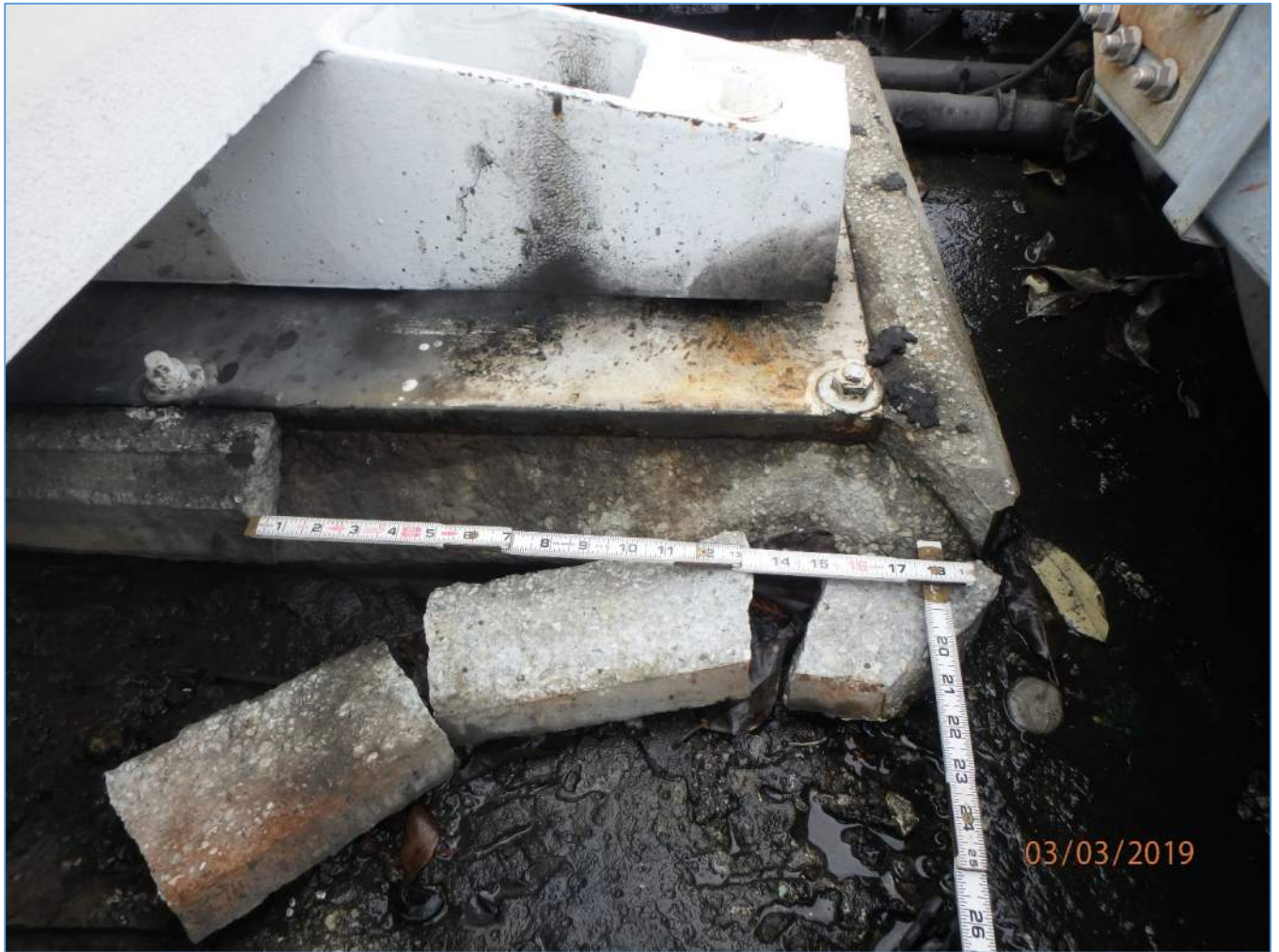
Span 31S: Switchbeam Pedestal Fractures and Spalls
