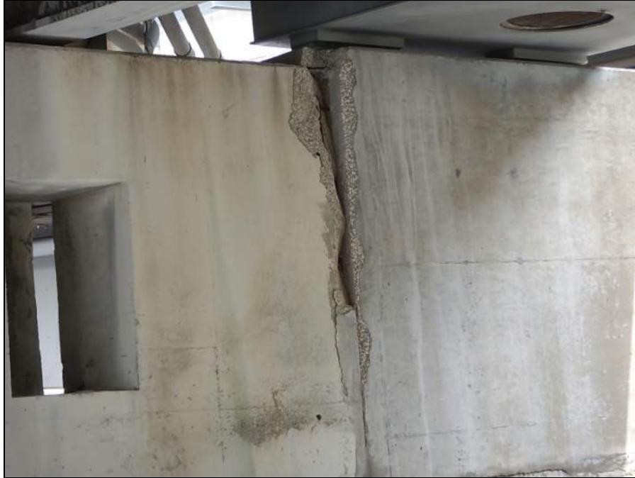
PHOTO 21 – ELEMENT 234 (W.O) VIEW OF 69 IN. X 17 IN. X UP TO 3 IN. DEEP SPALLED AREA IN SOUTH FACE OF PIER CAP 1, ADJACENT TO MONORAIL SKYWAY EXPRESS
