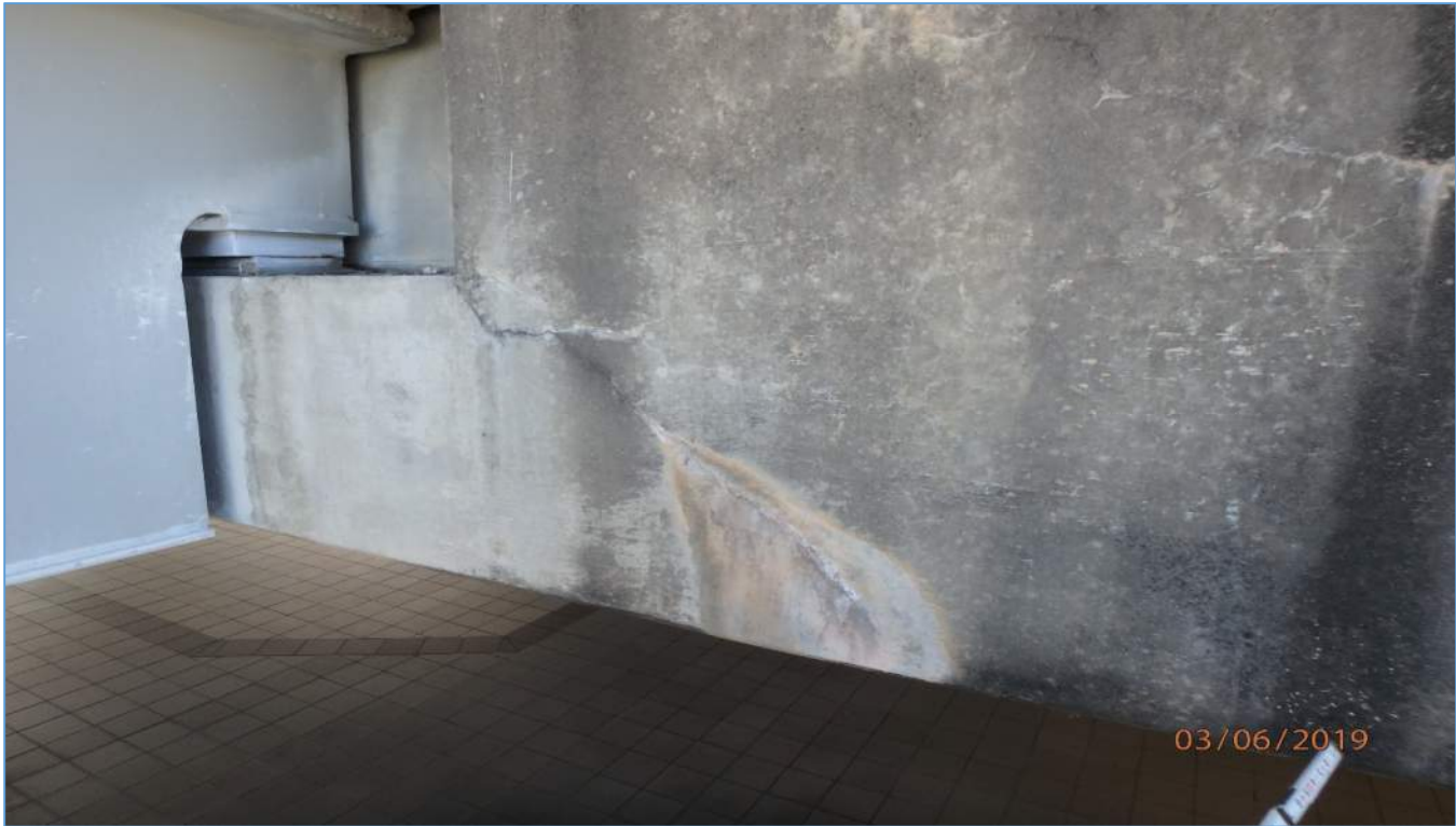
Pier 240: Diagonal Shear Cracks on the Front Face near the LT Column
