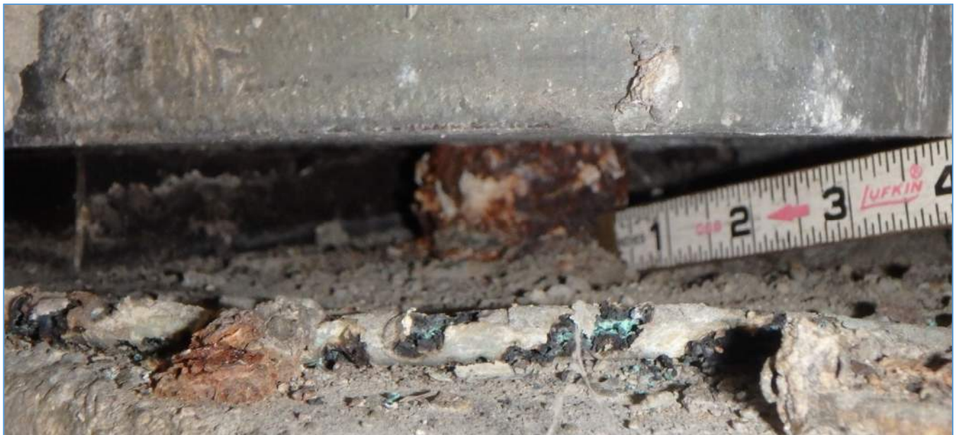
Span 239L at Pier 240L: Surface Corrosion on Bearing Plate Anchor Bolt
