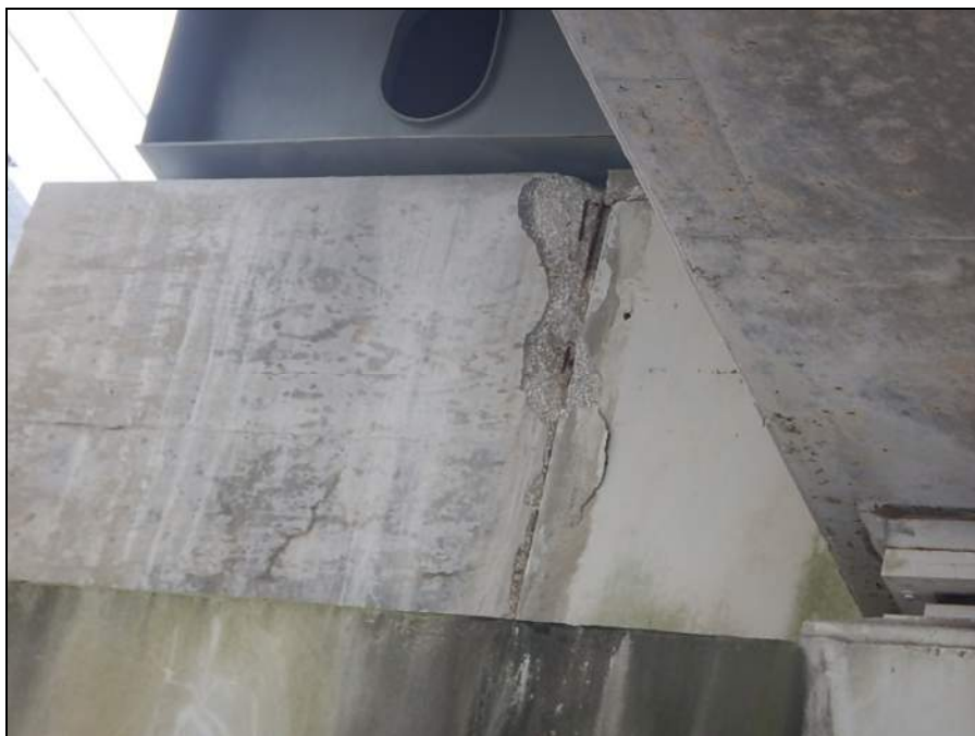
PHOTO 22 – ELEMENT 234 (W.O) VIEW OF 92 IN. X 15 IN. X 5 IN. DEEP SPALLED AREA IN NORTH FACE OF PIER CAP 1, ADJACENT TO MONORAIL SKYWAY EXPRESS
