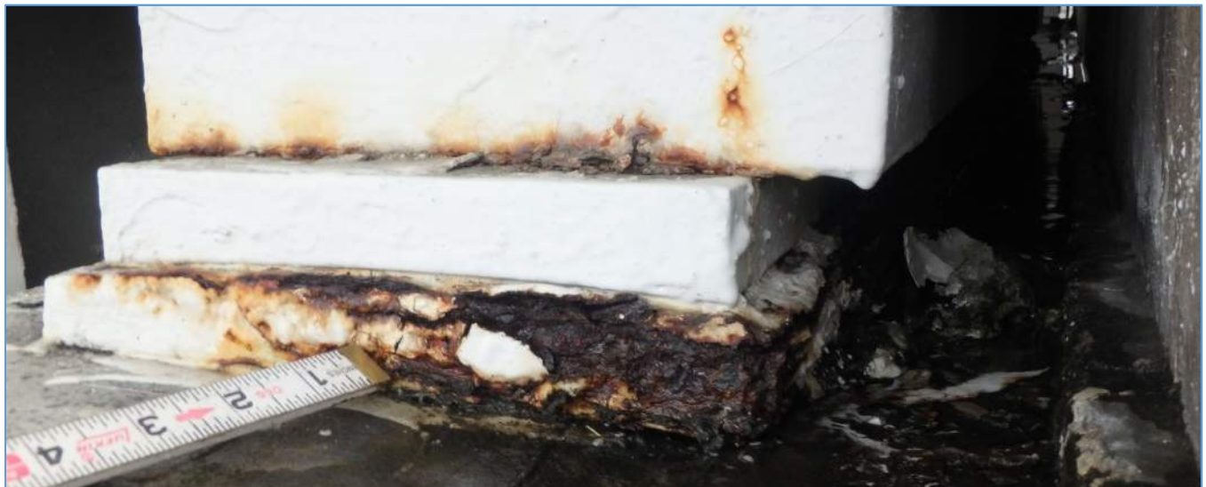
Span 29N at Pier 29N: Heavy Surface and Laminating Corrosion on Bearing Plates
