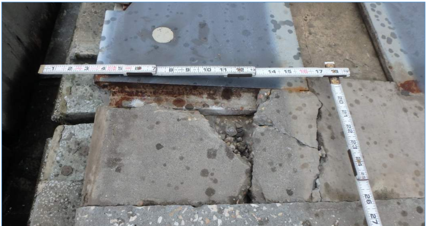
Pier 29N: Spalling and Delaminations on Forward Pourback
