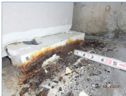
Keeper Plate with Corrosion
