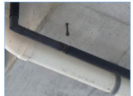
Broken Pipe Hanger Due To Surface Corrosion in Span 1N
