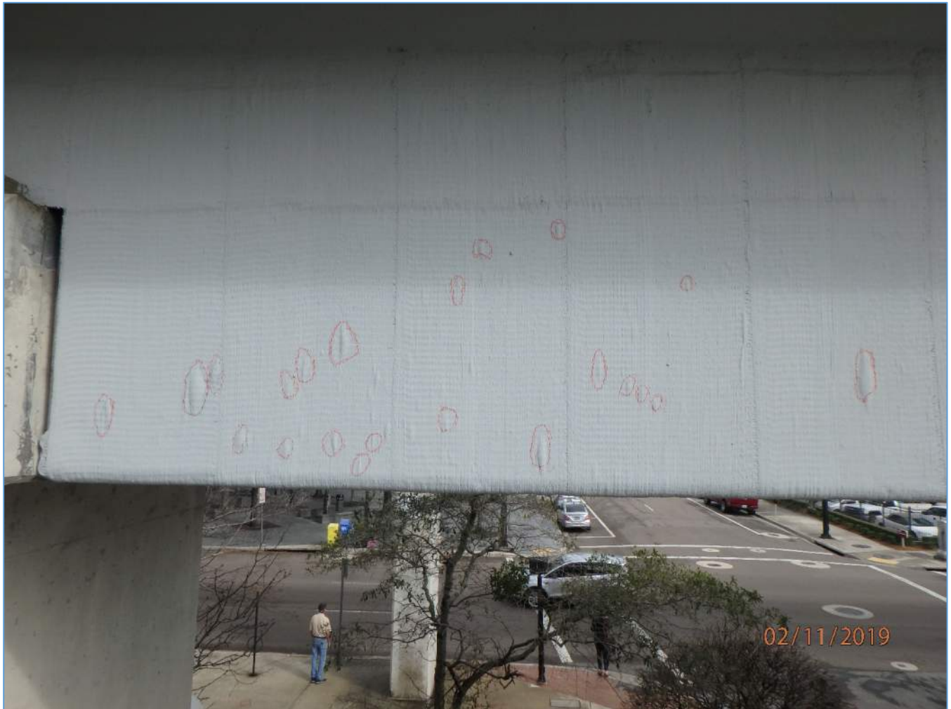
Span 47R: Delaminated Blisters on CFRP Wrap, Right Stem at Pier 47R
