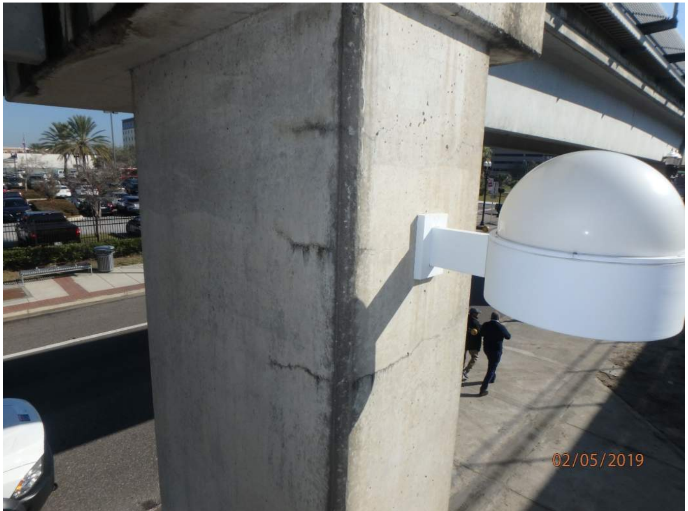
Pier 25N: Horizontal Flexure Cracking in Column with Cantilever Cap
