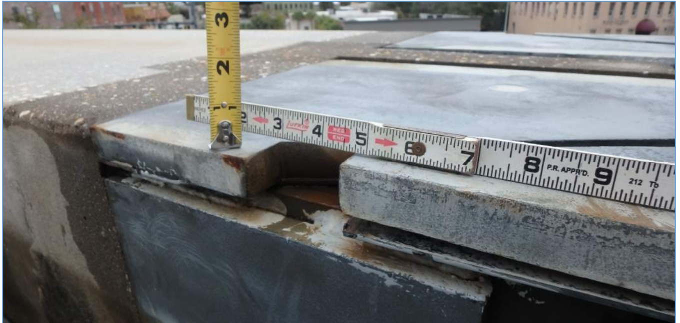
Pier 210L: 1/2" Elevation Difference Between Guidebeam Sliding Plates
