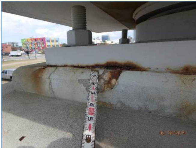
Pier 10: Surface Corrosion on Bearing Plate
