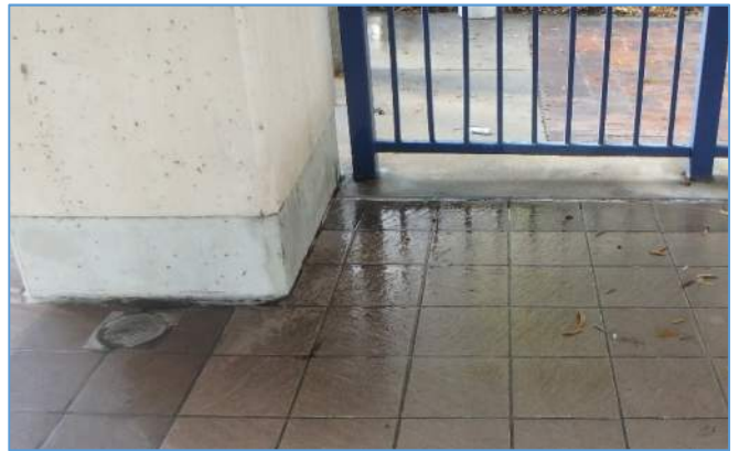
Pier 44S: Wet station tile due to failed deck joint
