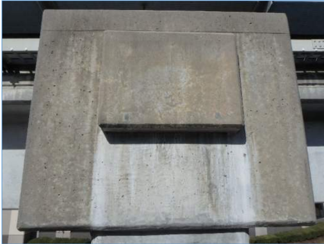
Pier 20N: Efflorescence Leaching from PT Cover
