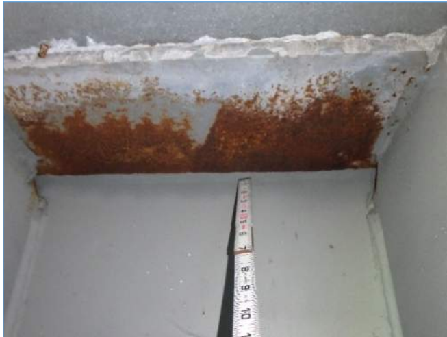
Span 408L: Corrosion on Top Flange at Bearing
