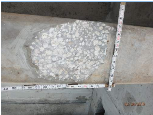
Span 75R: Looking Up at 10-1/2" x 9" x 1-1/2" Spall, Left Stem Near Pier 76R
