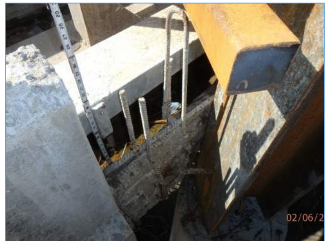
Span 5N: Sidewall Cutout at the JRTC Due to Conflict with Adjacent Building Column
