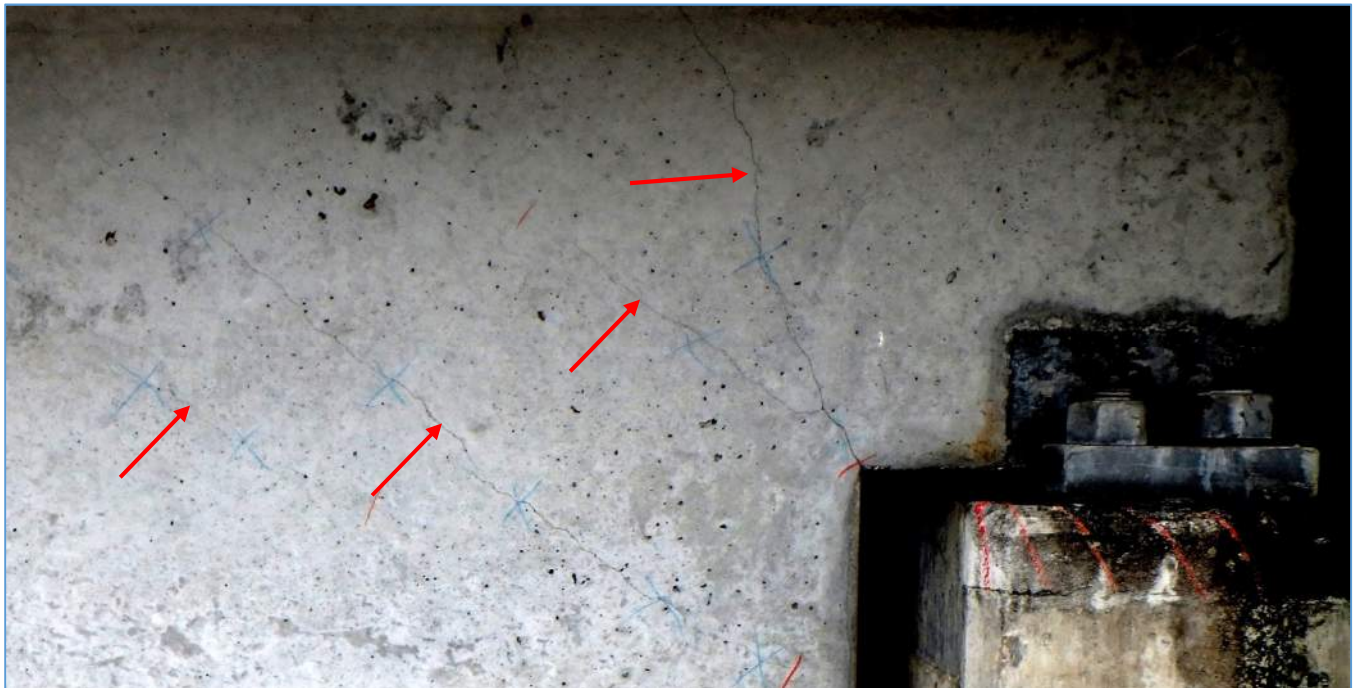
Span 12N: Shear Cracking up to 0.02" Wide on Left Stem End at Pier 12
