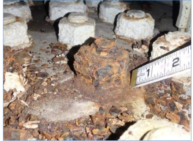
Span 52A LT, Bay 1 Splice (Up to 20% Loss on Nuts)
