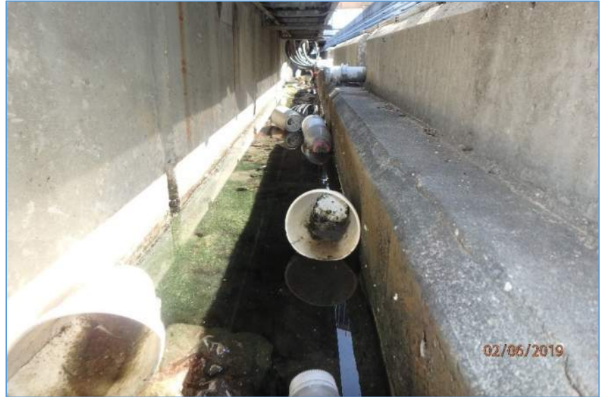
Span 2N: Trash, Debris and Standing Water
