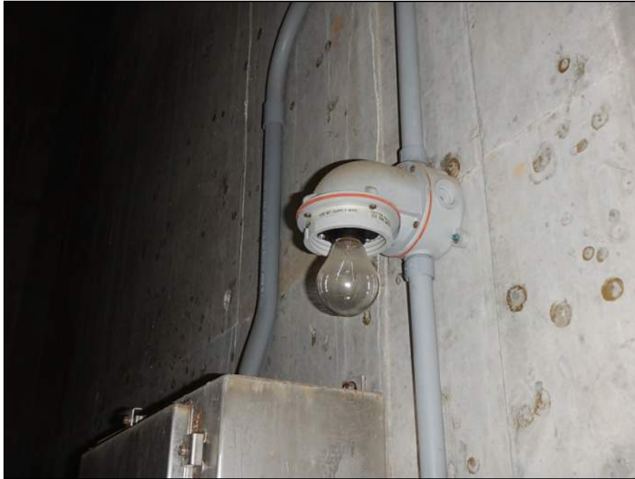
PHOTO 19 – ELEMENT 210 TYPICAL VIEW OF THE GLASS LIGHT LENS COVERS MISSING IN PIER 6
