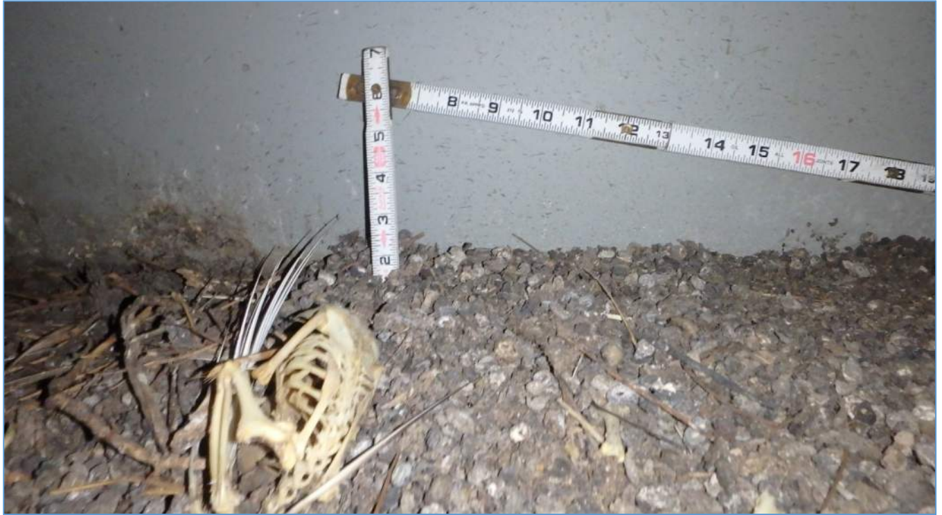
Span R6 LT: Organic Debris up to 2" Deep
