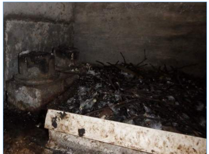
Pier 44: Wet Debris and Nesting Material on Cap
