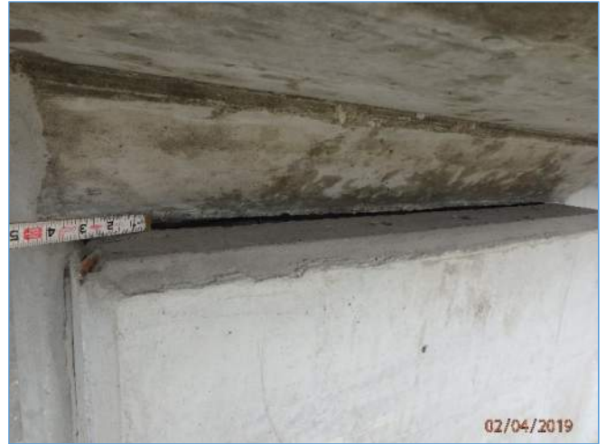
Pier 14N: 3/8" Gap at Top of PT Cover and Failed Caulk
