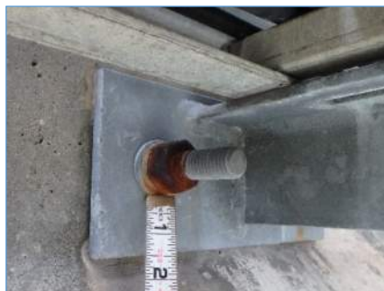
Corrosion on Nuts for Cable Tray Brackets, Starter Line
