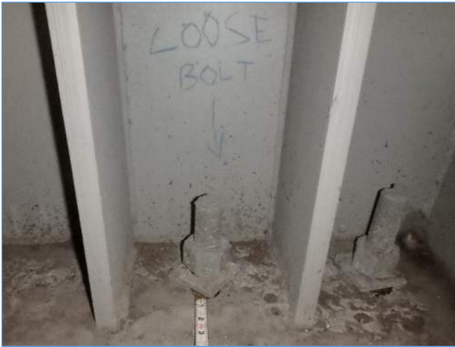
Pier R6: Loose Anchor Bolt and missing Jam Nuts
