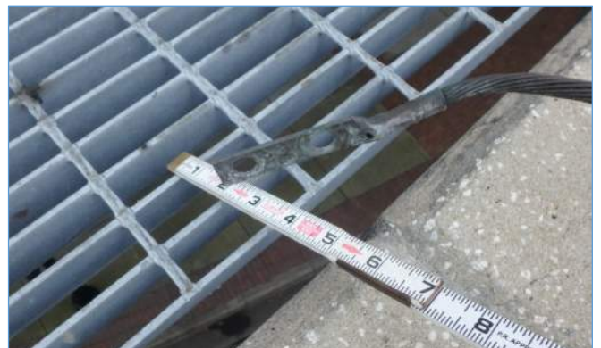
Span 78L: Detached Emergency Walkway Ground Wire
