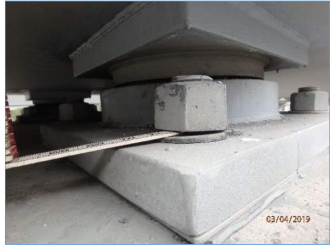
Pier 256L: Loose Bearing Anchor Bolt Nuts
