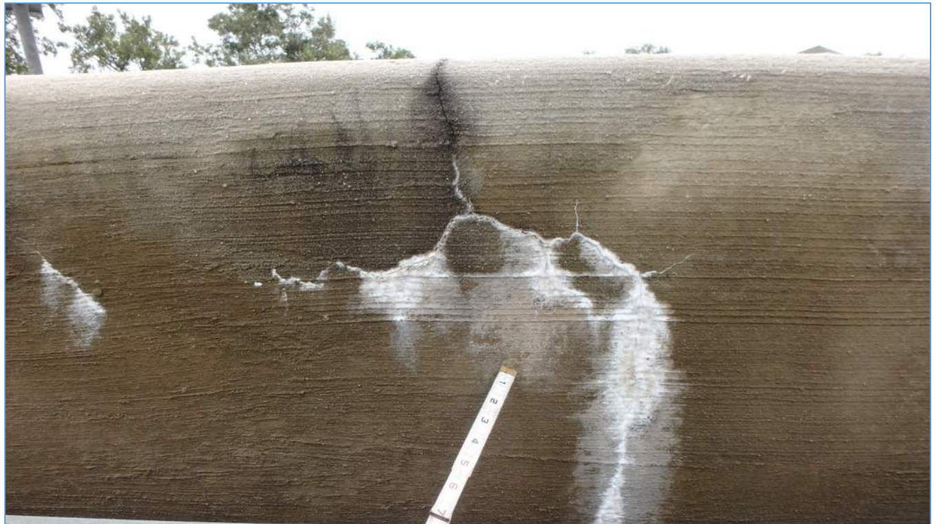
Span 211L: Random Cracking on the Interior Face of the Left Sidewall with Efflorescence
