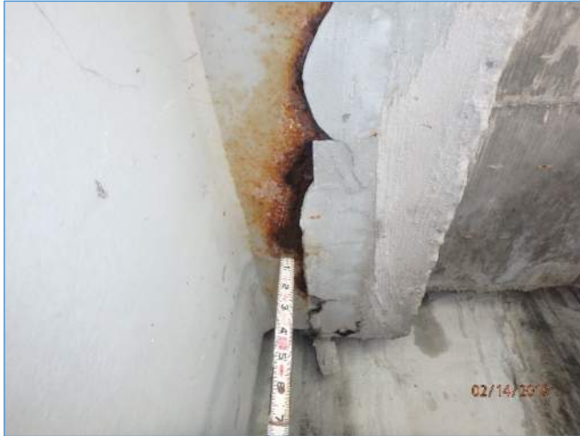
Span 236L: Surface Corrosion on RT Top Flange
