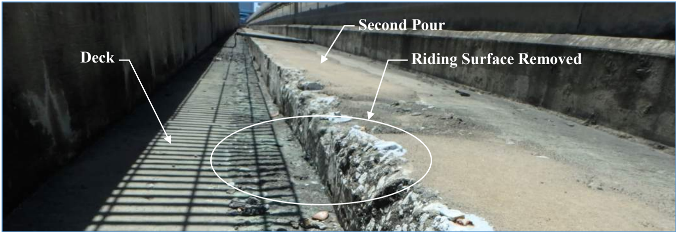
Typical Deck Top in the Starter and North Lines Showing Removal of Relic Riding Surface (Photo from 2017)
