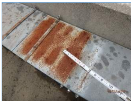
Surface Corrosion on Cable Tray Top in Span 29N
