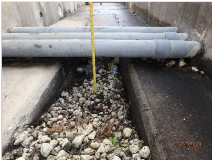
Erosion Between Slab-on-Grade Spans at the O&M Center
