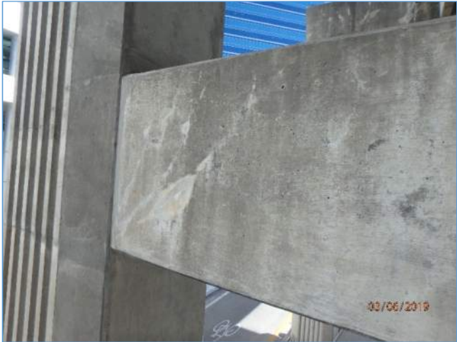
Pier 238: Diagonal Shear Cracks on Strut at RT Column
