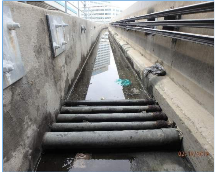
Pier 240R: Standing Water Blocked by Conduits
