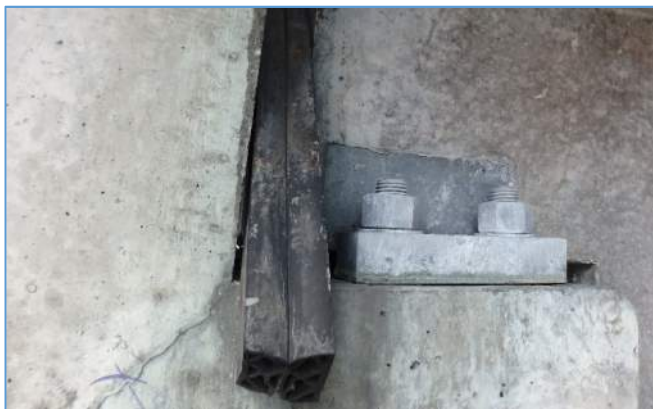
Pier 81L: Joint Seal Hanging Down
