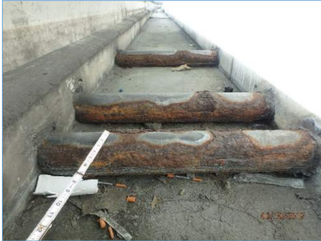
Pier 239L: Heavy Surface Corrosion on Conduits
