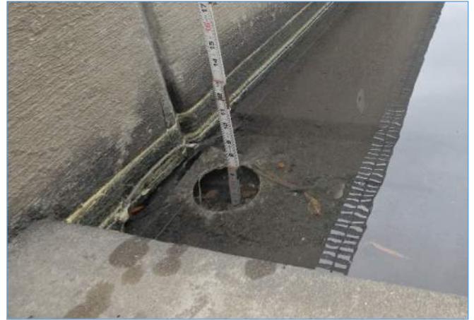
Span 244R: Missing Atrium Grate and Drain Pipe Clogged and Filled with Water
