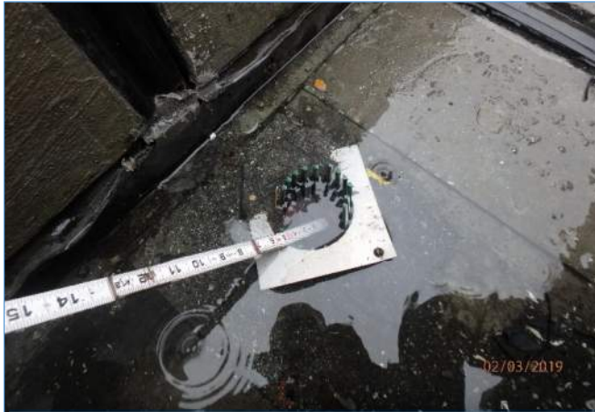
Pier 219R: Broken Atrium Grate and Drain Pipe Clogged and Filled with Water
