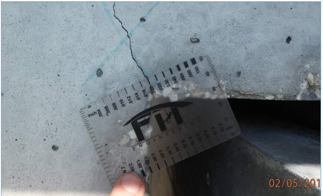
Span 12N: Close-up of Shear Crack in Left Stem at Pier 12
