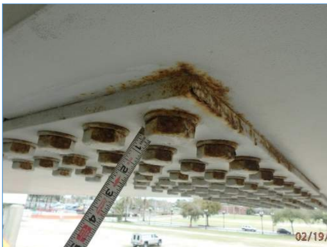
Span 10N: Corrosion on Splice Plates and Bolts
