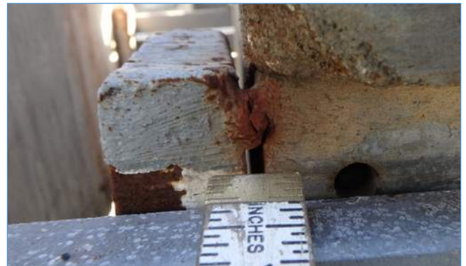
Pier R-6R: Retrofit Plate Tack Weld Crack
