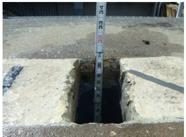
Span 2N: Water Inside Guidebeam
