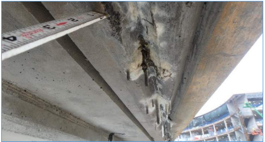
Span 8N: Heavy Efflorescence and Moisture Leaching in Deck Overhang
