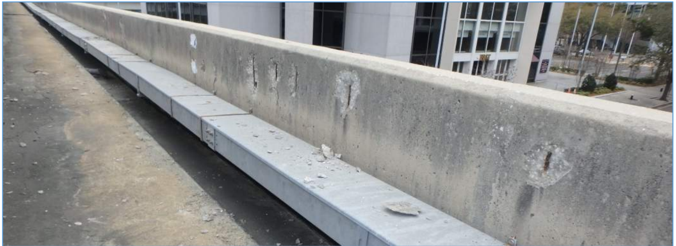
Span 55L: Interior Face of Left Sidewall with Insufficient Reinforcement Cover Spalls
