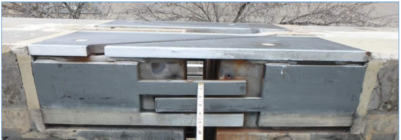
Pier 78L: Missing Finger on the Right Side of the Guidebeam
