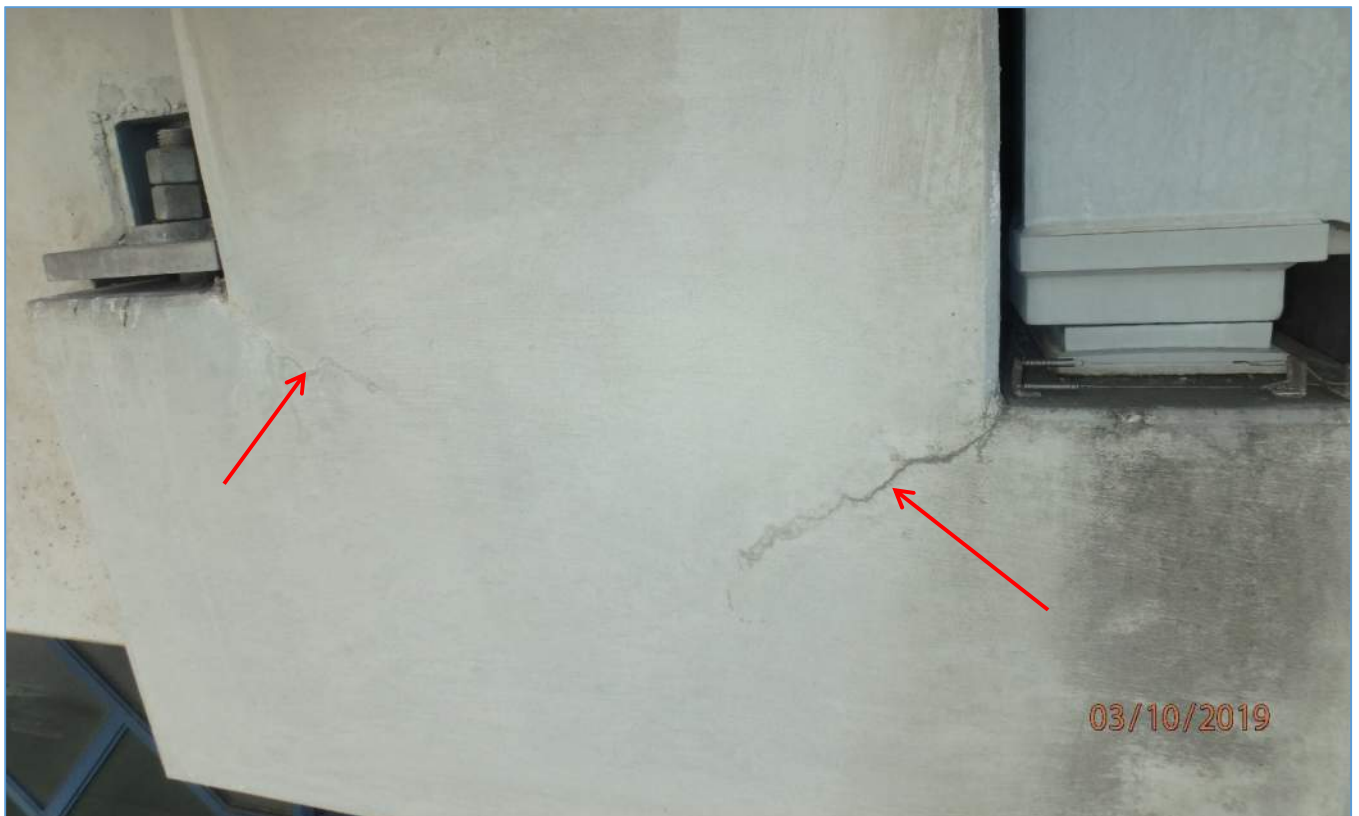
Pier 240, Right Face of Cap: Typical Beam Seat Corner Cracks
