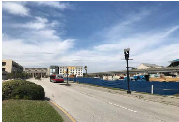
Looking west toward Jefferson Station at Lofts of LaVilla construction. Completed Fall 2017.
