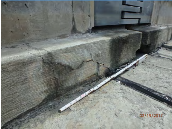
Pier 207: Guidebeam Pedestal Cracking
