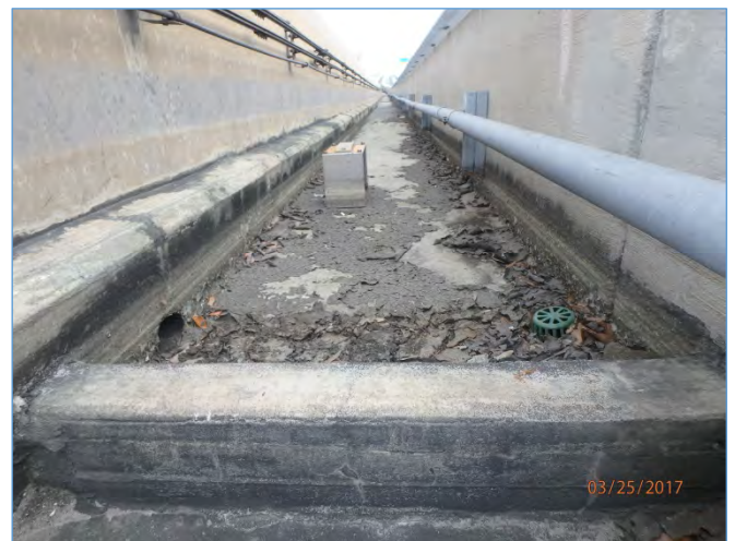
Span 245L After Partial Debris Removal
