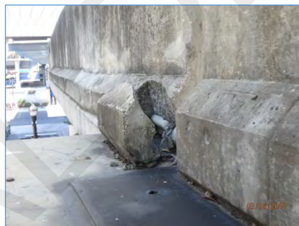
12in. x 6in. x 6in. Spall in Sidewall Bottom Edge Over Pier 78
