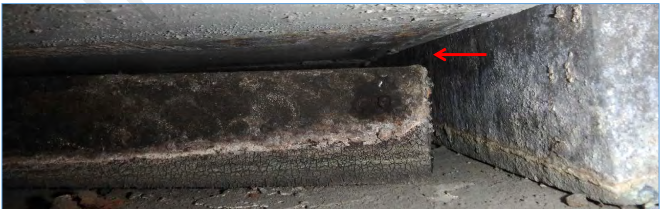
Span 202R: 1/4" Gap Between Left Stem and Bearing Pad at Pier 202R
