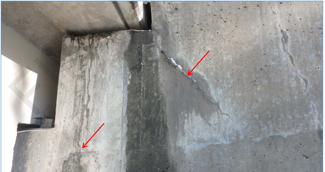
Pier 62: Diagonal cracks extending downward from the left beam seat corner and the top flange notch.
