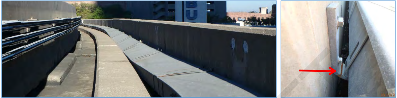
Span 55L Cable Tray with Three Broken Attachment Brackets
