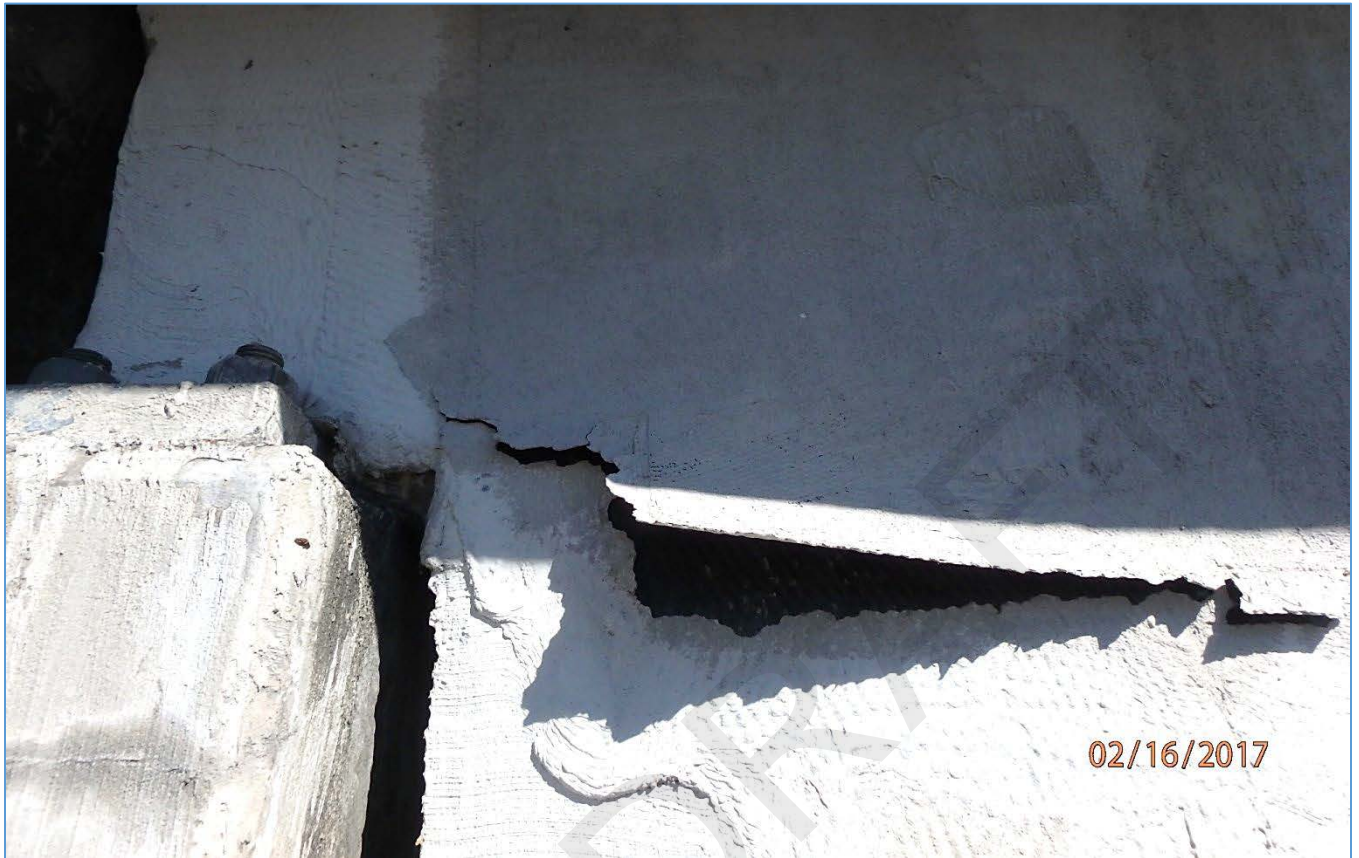
Span 227L: CFRP Failure in at Pier 228
