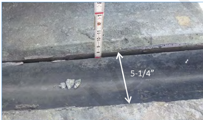
Pier 232R: Joint Width Exceeds Seal Capacity
