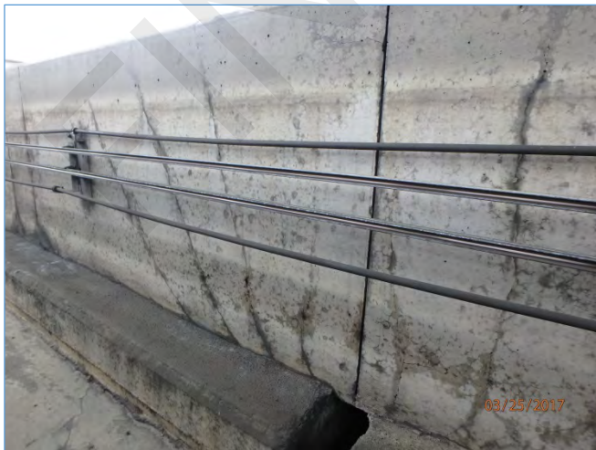
Span 253: Vertical Cracking in Guidebeam
