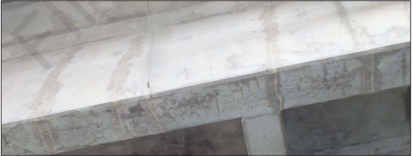
Span 42S – Cross: Typical Sealed Flexural Cracking in Beam Stems
