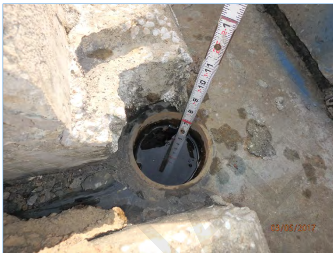
Missing Cap and Clogged Pipe at Pier 12, LT Guideway
