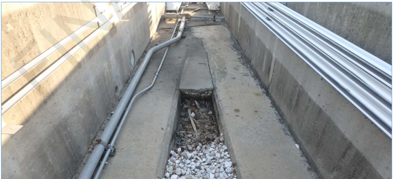
Erosion Between Slab-on-Grade Spans M1B3 and M1B4 at the O&M Center
