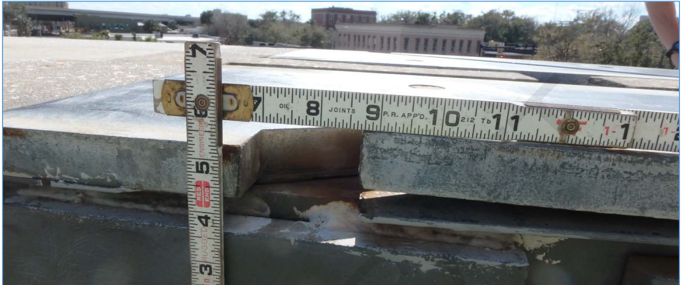
Pier 210L: 1/2" Elevation Difference Between Guidebeam Sliding Plates
