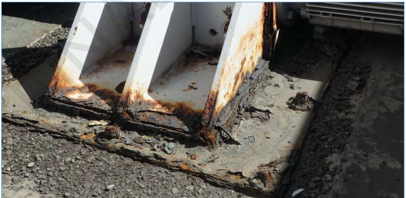
Span 213L: Surface Corrosion and Section Loss on Switchbeam Machinery Support Brackets
