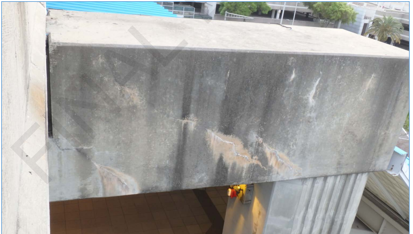
Pier 240: Diagonal Shear Cracks on the Front Face near the LT Column
