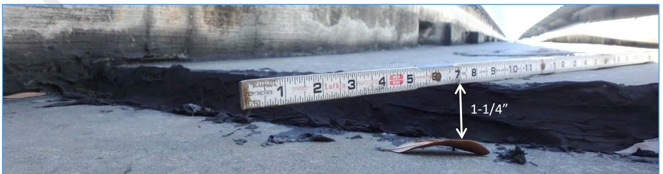
Pier 228R: 1-1/4" Elevation Difference Between Top of Deck and Top of Pier Cap
