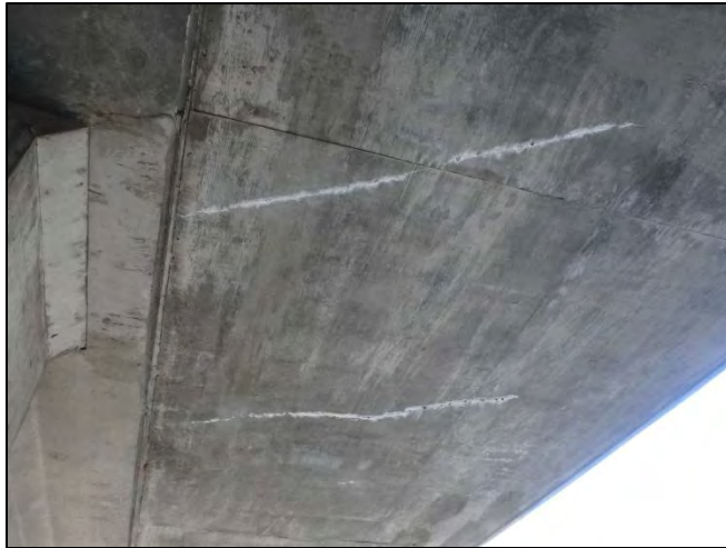
Span 75R: Transverse Cracking on the CIP Deck Underside
