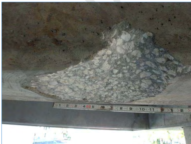
Span 75R: 10-1/2"x9"x1-1/2" Spall, Left Stem Near Pier 76R
