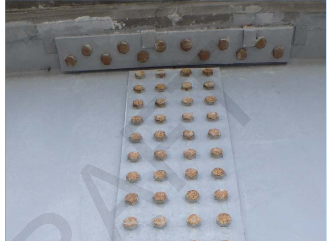
Span 405R: Surface Corrosion on Exterior Splice Bolts
