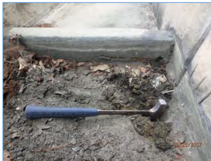
Missing Drain Cap and Clogged Pipe above Pier 255, RT Guideway
