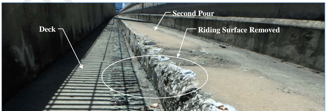
Typical Deck Top in the Starter and North Lines Showing Removal of Relic Riding Surface
