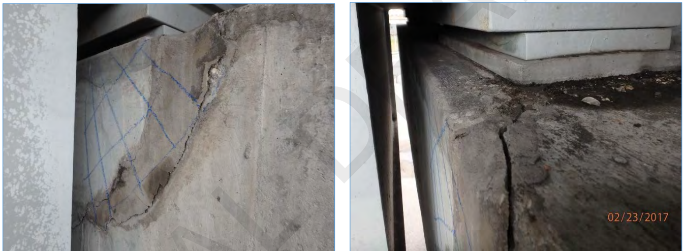
Pier 258R: Large Delamination Below the Right Bearing, Rear Face
