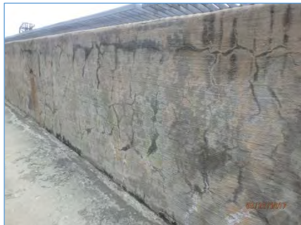
Hairline Map Cracking for 10ft., Span 250R
