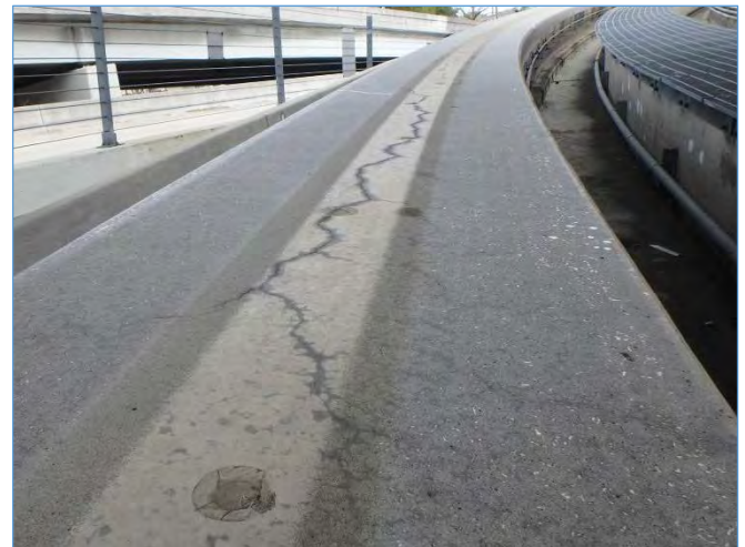
Span 253: Longitudinal Cracking in Guidebeam
