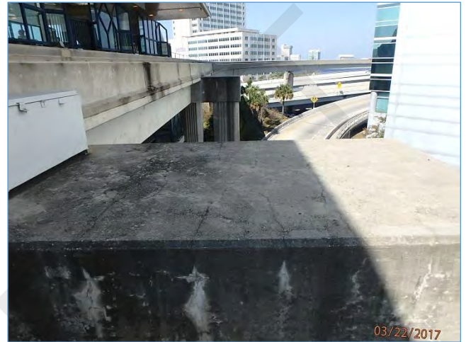
Pier 238: Flexure/Shear Cracks Across Cap at RT Column
