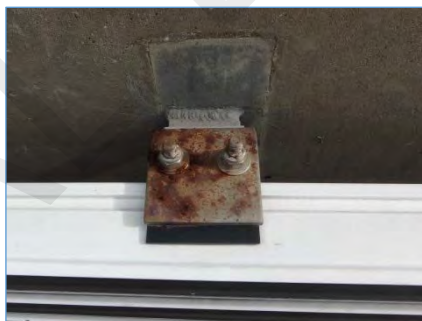
Surface Corrosion on Power Rail Bracket in Span 206R
