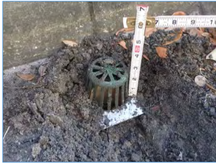
Buried Drain Cap at Pier 247, LT Guideway
