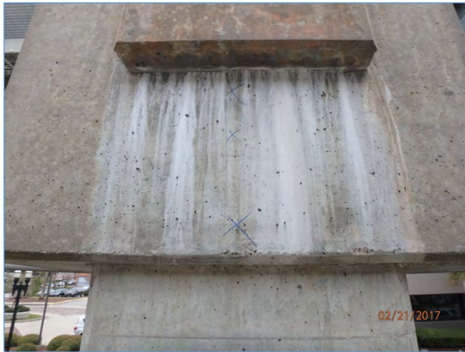
Pier 19N: Efflorescence Leaching from PT Cover
