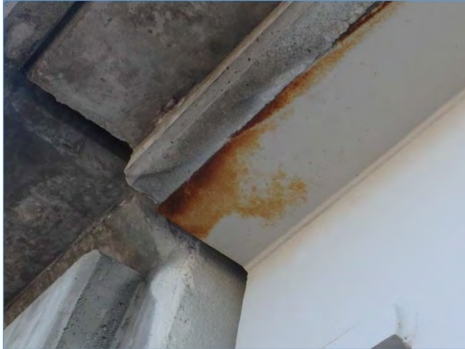
Span 31N: Surface Corrosion on LT Top Flange
