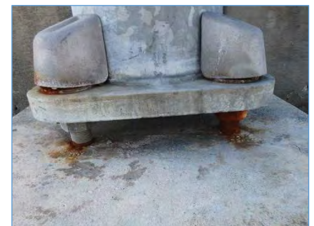
Surface Corrosion on Traffic Signal Post Anchor Bolts in Span M2.
