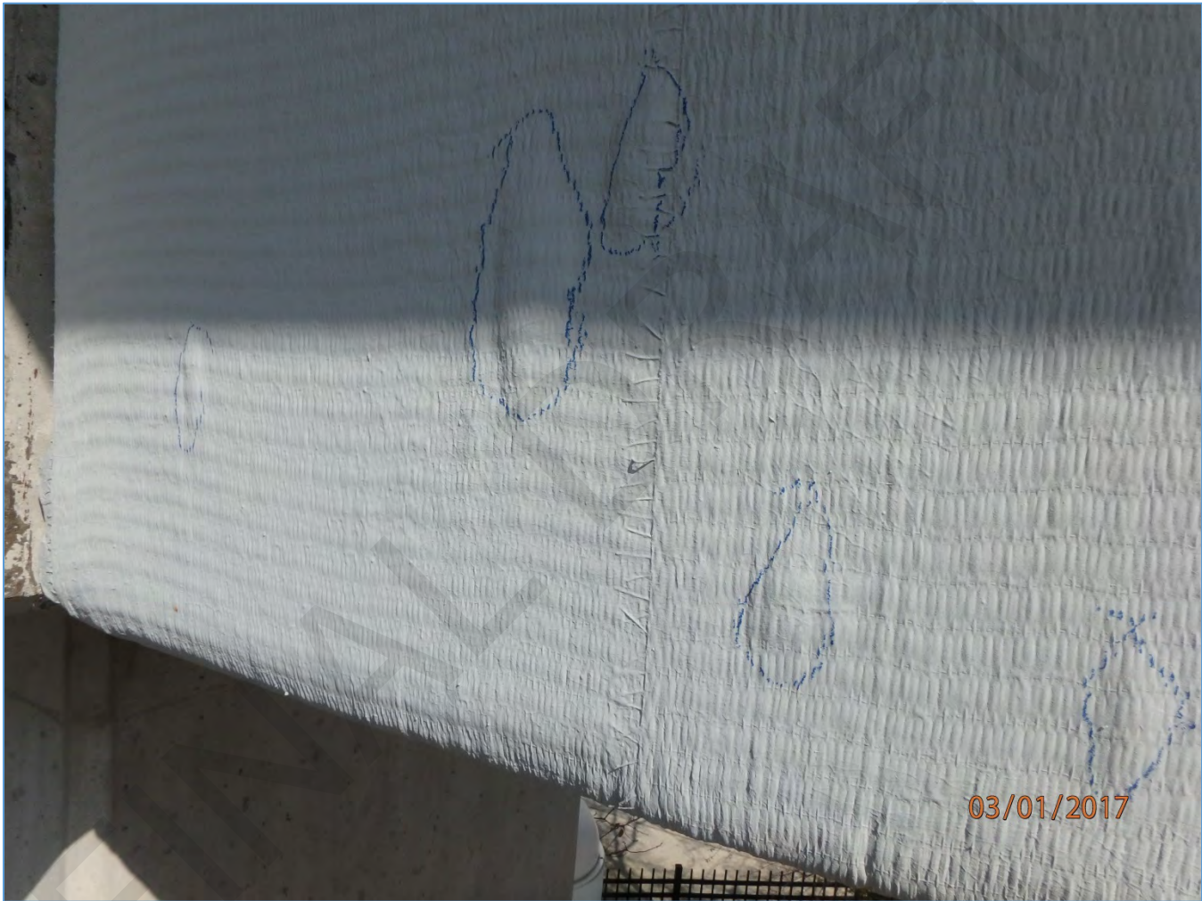
Span 47R: Delaminated Blisters on CFRP Wrap, Right Stem at Pier 47R
