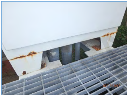
Surface Corrosion on Electrical Control Cabinet in Span 204R
