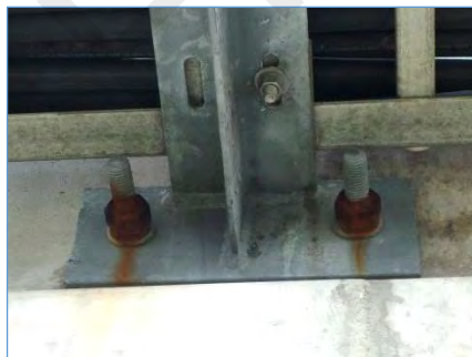
Non-galvanized Nuts for Cable Tray Brackets, Starter Line
