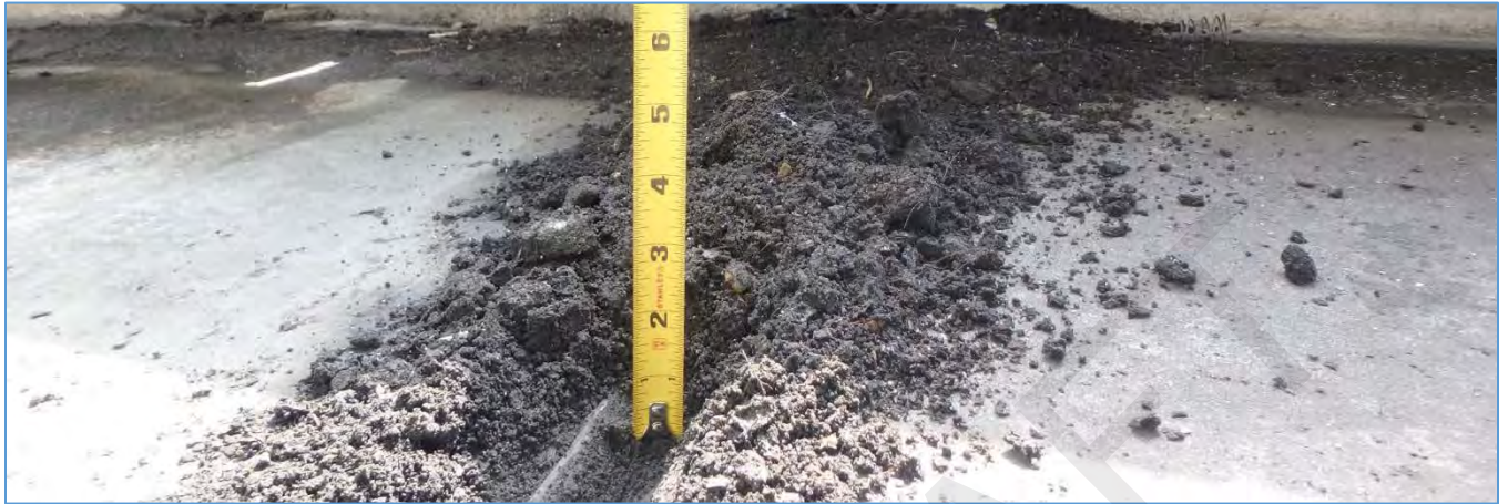
Pier 223L: 1-1/4" Joint filled with soil and debris.
