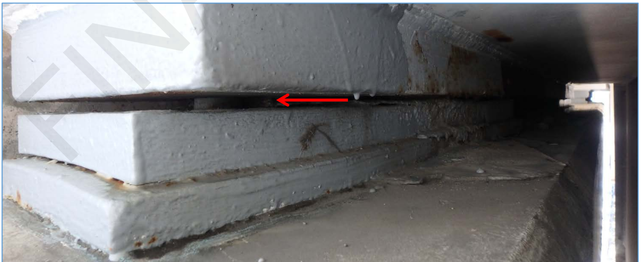
Span 52A Left at Pier 52A: 1/4" Gap Between Sole Plate and Bronze Plate
