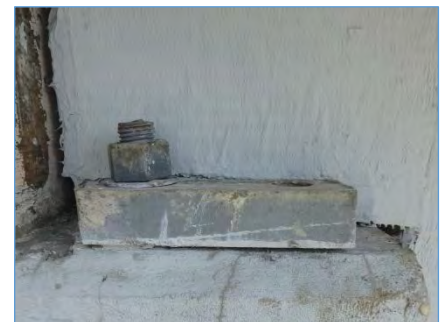
Keeper Plate Missing Anchor Bolt
