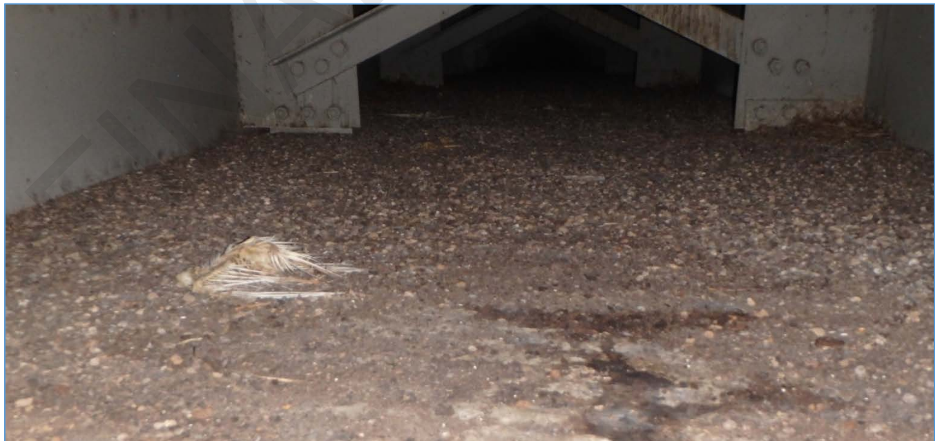
Span R-6 LT: Organic Debris up to 2" Deep
