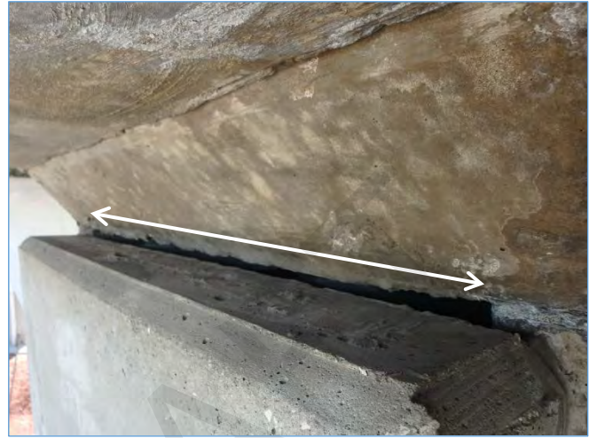
Pier 40N: 1/2" Gap at Top of PT Cover and Failed Caulk
