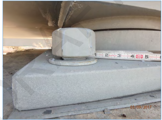
Pier 409L: Loose Bearing Anchor Bolt Nuts
