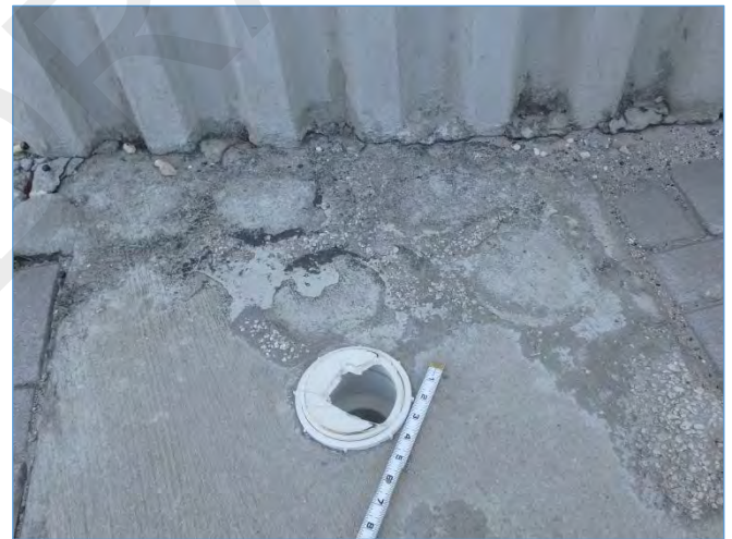
Broken Riser Pipe Cap at Pier 256L
