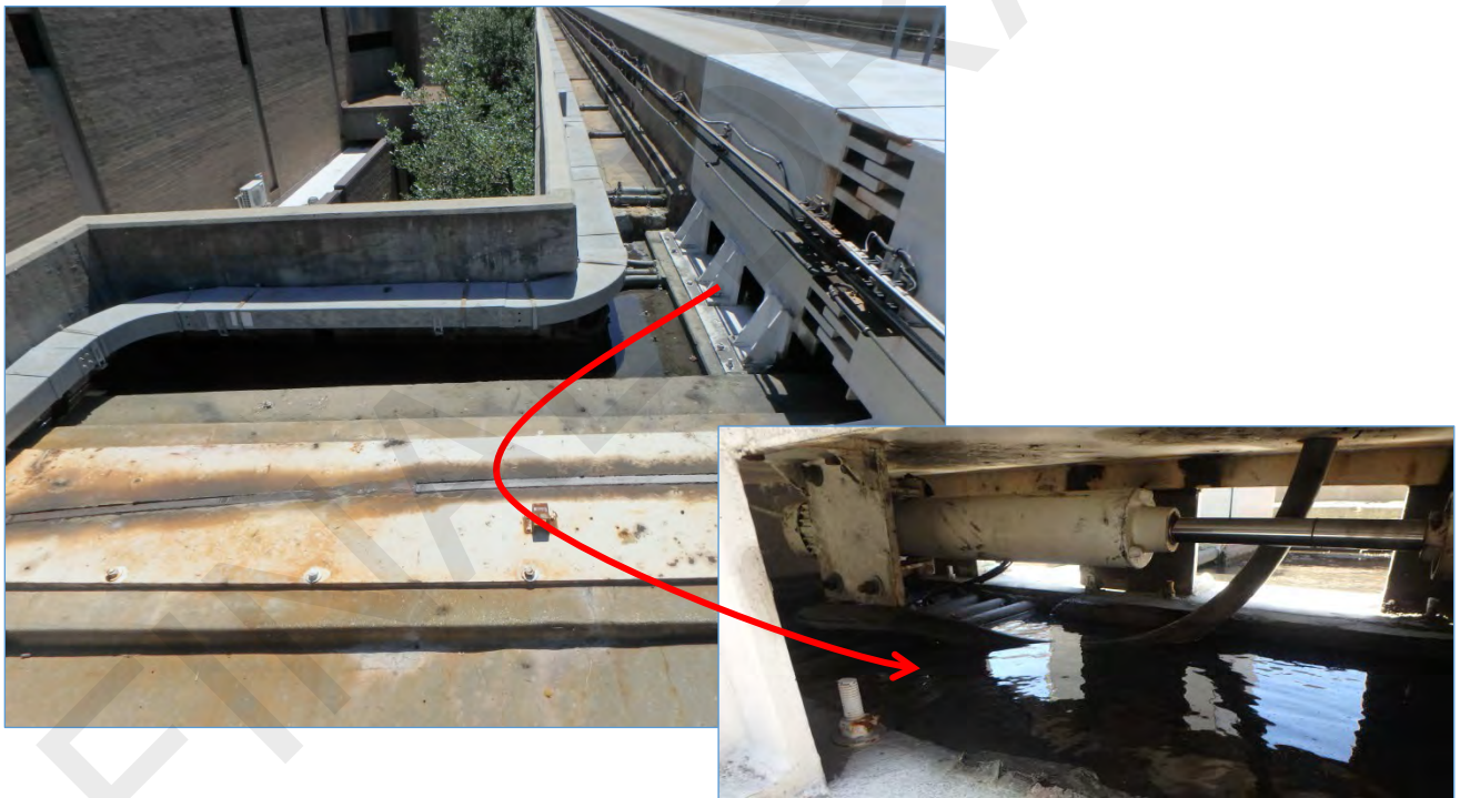
Span 75R Before Pier 76, Water Ponding Behind Switch Beam Pedestal #1 and Underneath Switch Beam
