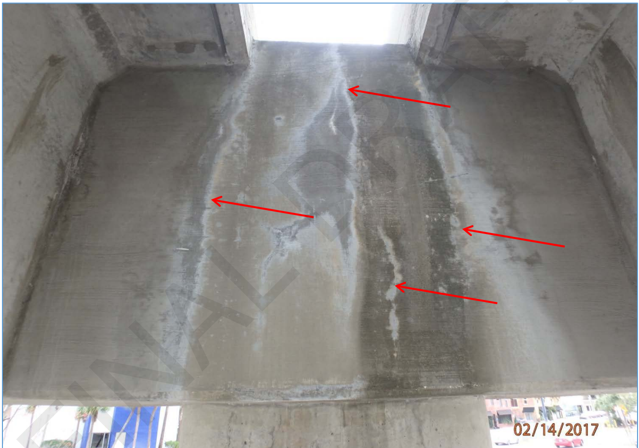
Typical Negative Moment Crack, Full Depth of Cap, Front Face of Pier 212
