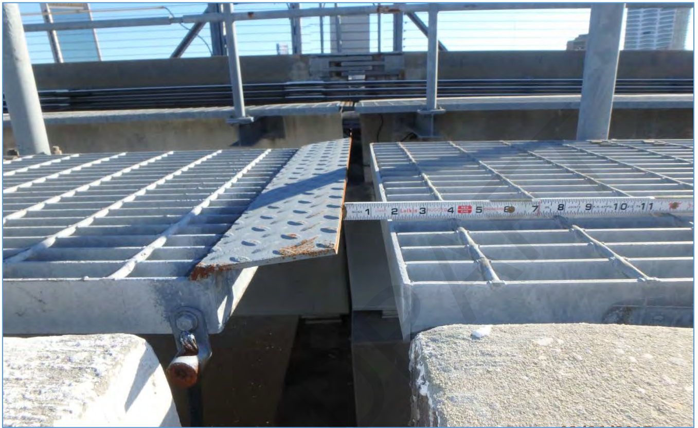
Pier R-1 LT, Emergency Walkway Joint Expanded Beyond Expansion Plate
