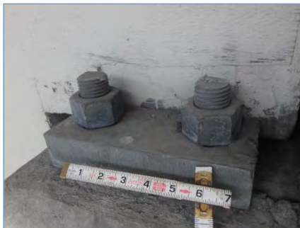
Keeper Plate Nut Missing Washer
