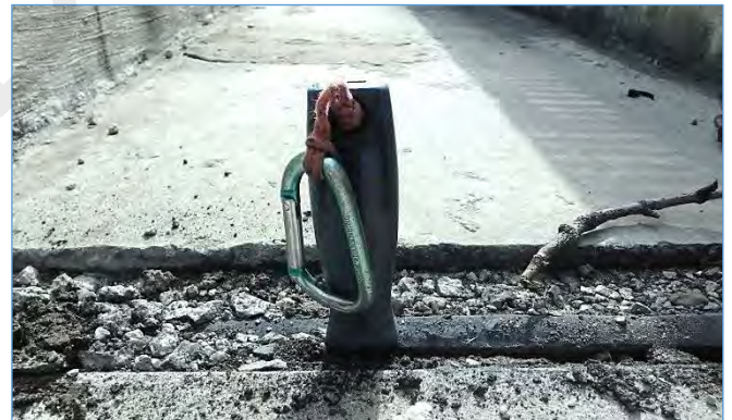
Pier 210R: Typical Seal Adhesion Failure
