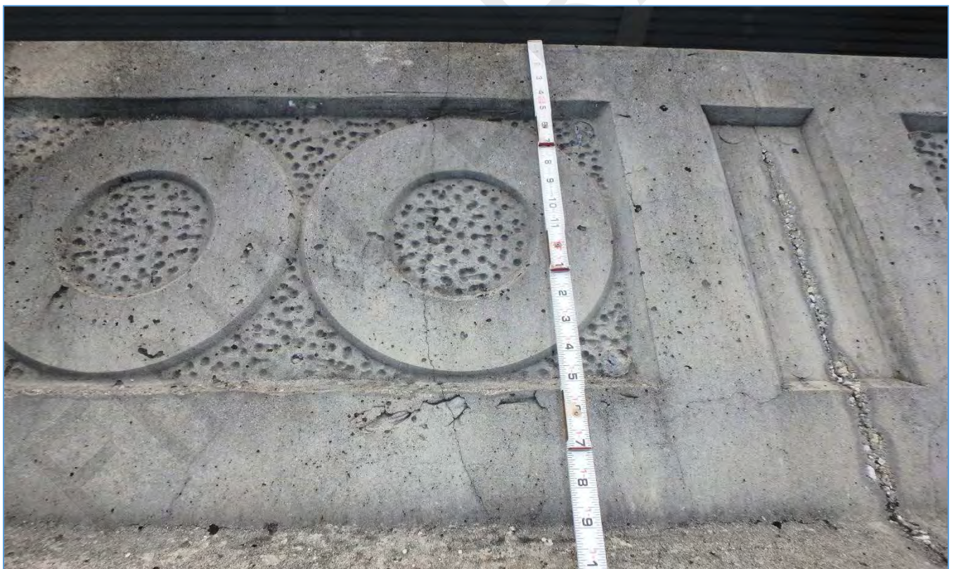
Typical Condition State 2 Cracking in the Sidewalls of the North Line
