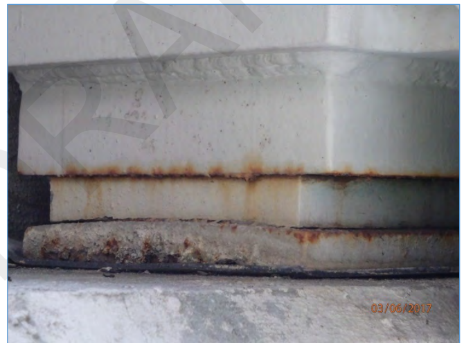
Span 206L at Pier 207L: Surface corrosion on Sole Plate and Masonry Plate
