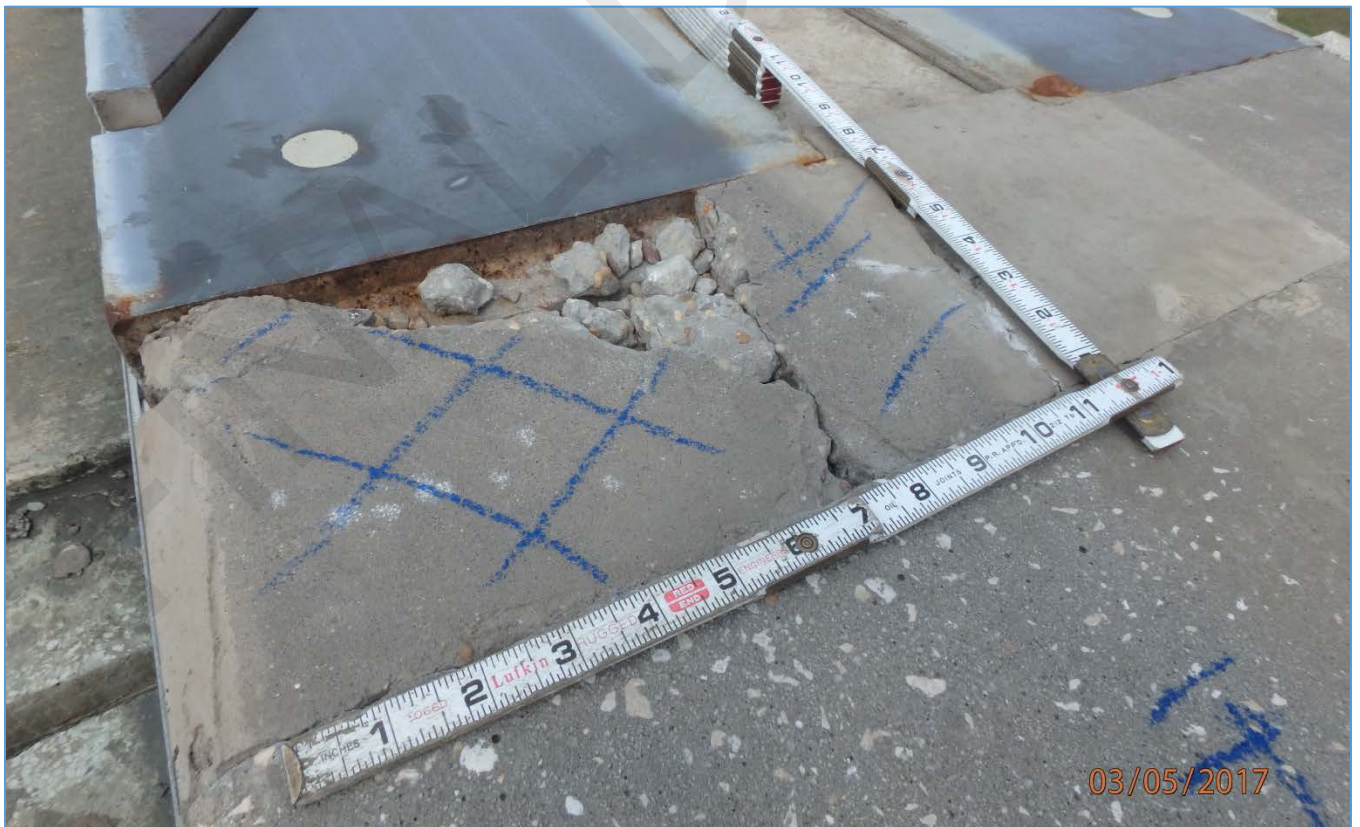
Pier 29N: Spalling and Delaminations on Forward Pourbacks
