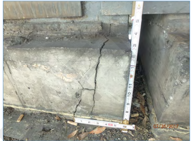
Pier 237: Guidebeam Pedestal Delamination
