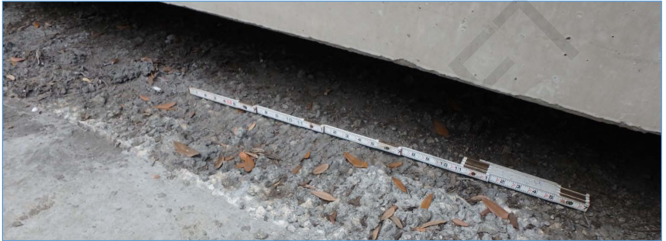
Typical Roughened Deck Top in the South Line Due to Intermittent Removal of Guidebeam Pedestal
