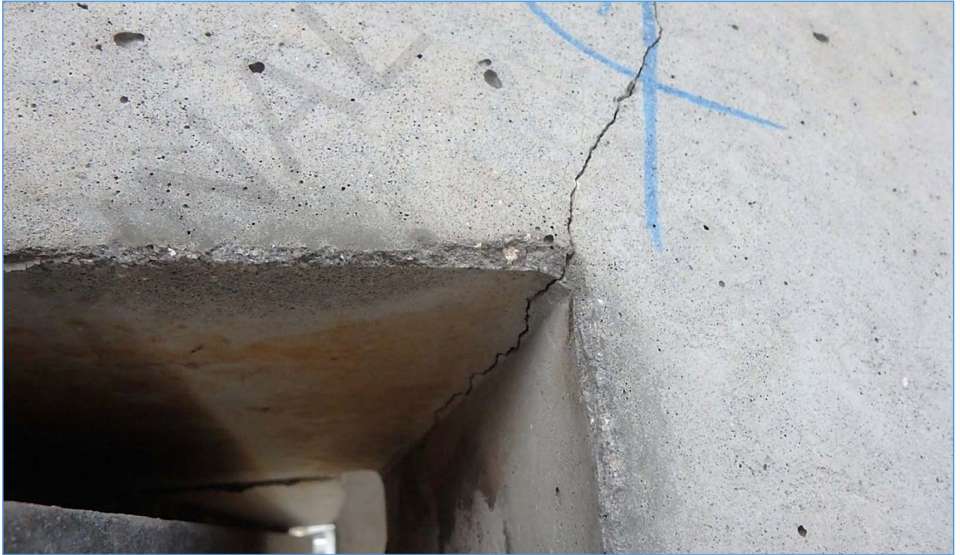
Span 24S: Full Depth Shear Cracking up to 0.03" Wide on Left Stem End at Pier 25S.
