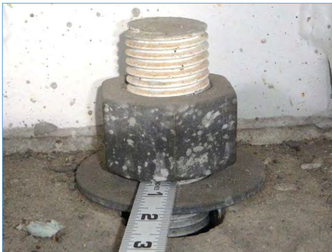
Span 205L at Pier 205L: Anchor Bolt Nuts Not Flush With Washers. Missing Jam Nuts.
