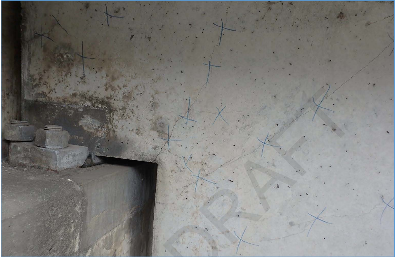
Span 18N: Shear Cracking up to 0.02" Wide on Right Stem End at Pier 18N.
