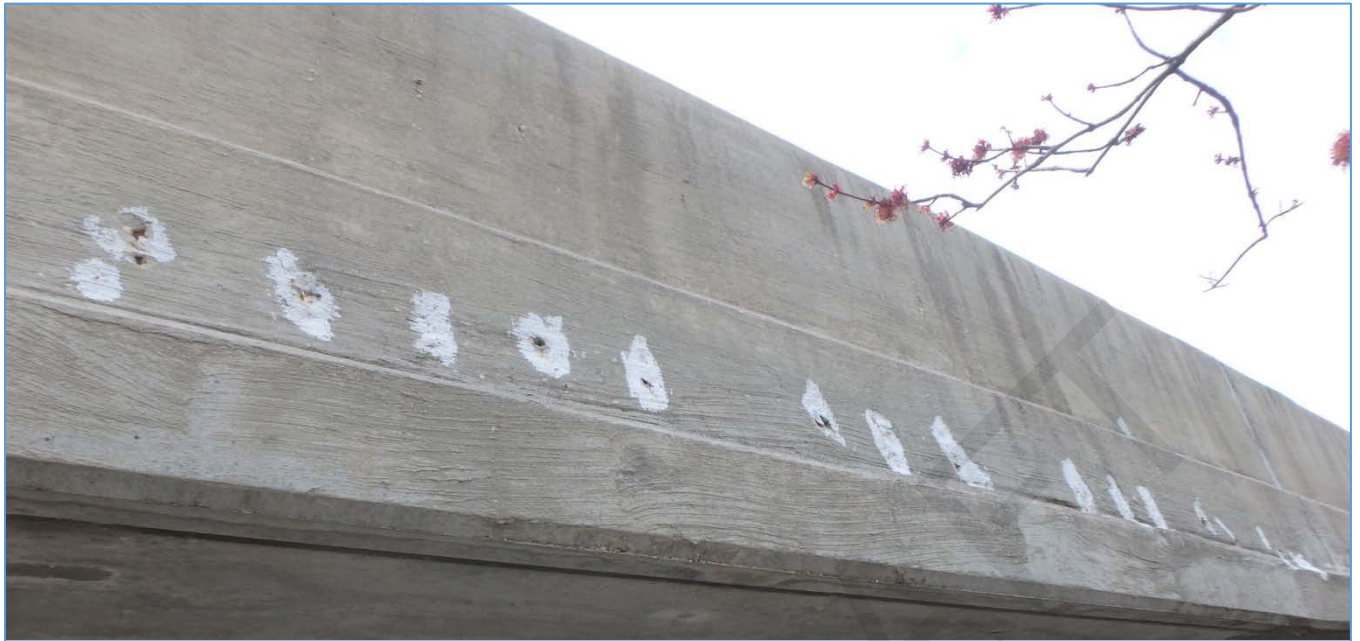
Shallow Spalls Due to Insufficient Cover in the Exterior Face of the Right Sidewall in Span 210R
