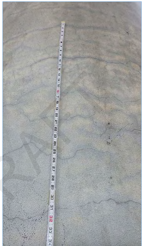
Close-up of Cracks
