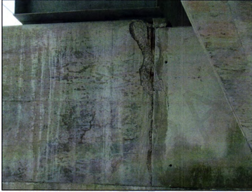
PHOTO 25 – ELEMENT 234 VIEW OF SPALLED AREA IN THE NORTH FACE OF PIER 1, UNDER THE PEOPLE MOVER
