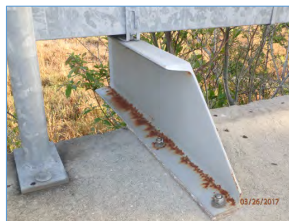
Surface Corrosion on Cable Tray Support Brackets in Span M2
