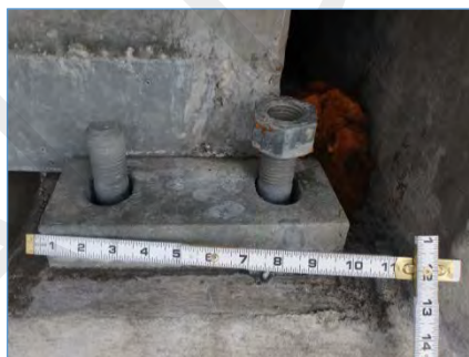
Keeper Plate Bolt Missing Nut
