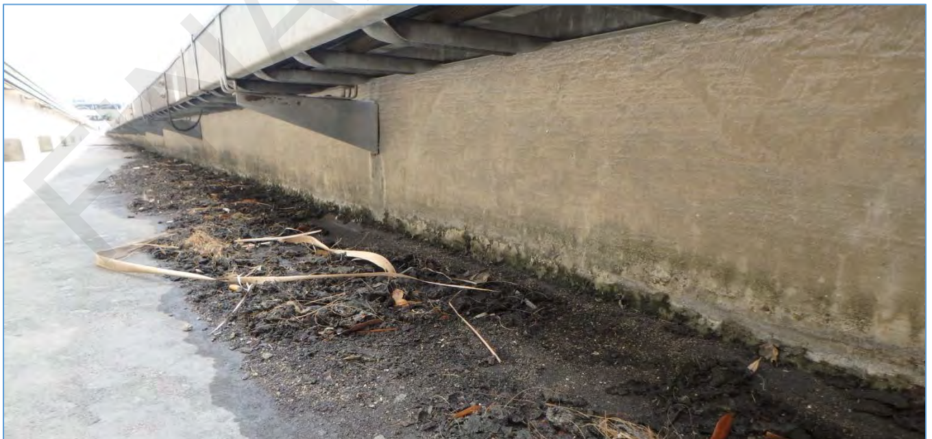
Span 213L: Wet Debris for 20' over Pier 214
