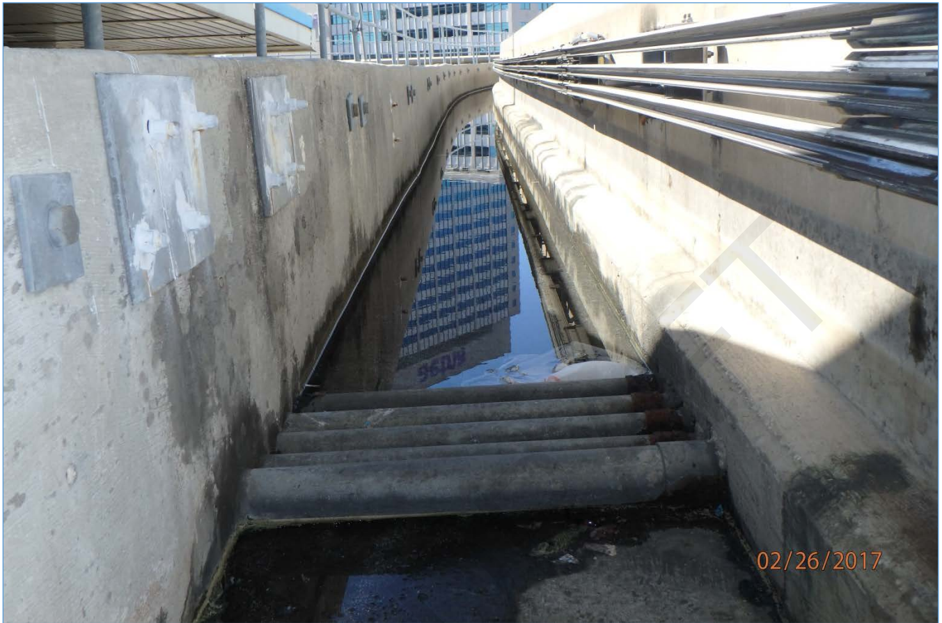
Span 240R: Ponding Water Left of the Guidebeam Blocked By Debris and Transverse Conduits on the Deck
