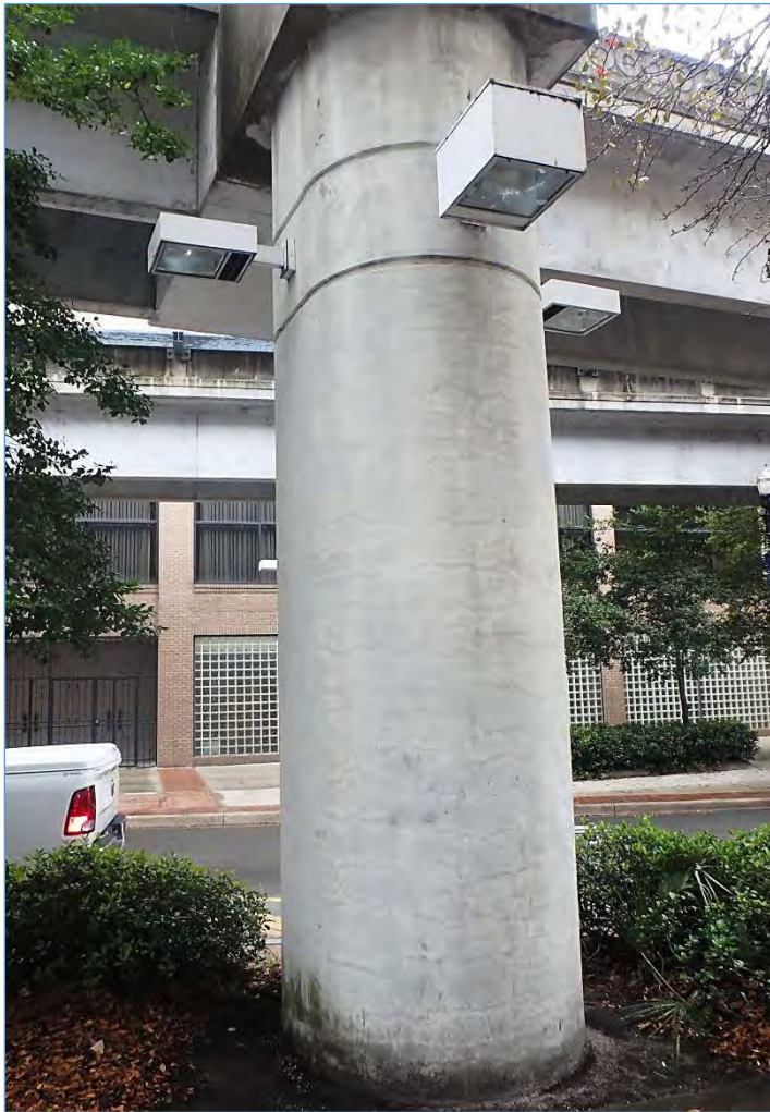
Pier 79R: Flexure Cracking in Column With Cantilever Cap
