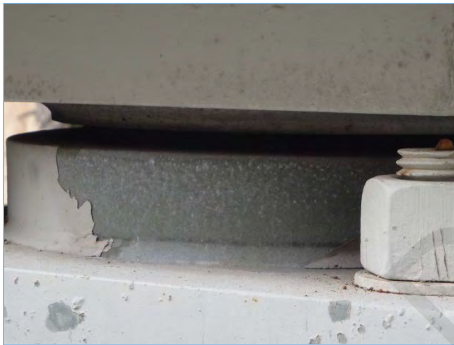
Pier 206L: Peeling Paint on Pot Bearing Cylinder
