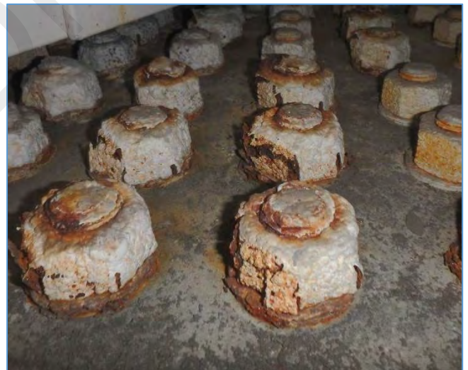
Span 52A LT, Bay 1 Splice (Up to 15% Loss on Nuts)
