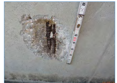
Spall with Exposed and Corroded Rebar, Span 5N
