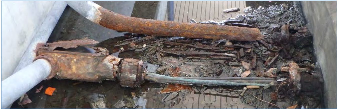
Span 238L – 100% Section Loss of Transverse Conduits, Exposing Wires
