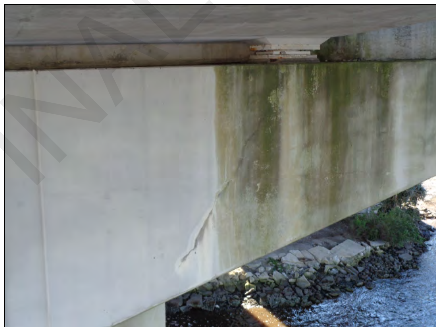
PHOTO 22 – ELEMENT 234 VIEW OF NORTH FACE OF PIER 1 CAP WHICH HAS INSIGNIFICANT HORIZONTAL AND DIAGONAL CRACKS WITH EFFLORESCENCE BELOW BEARING 1-1
