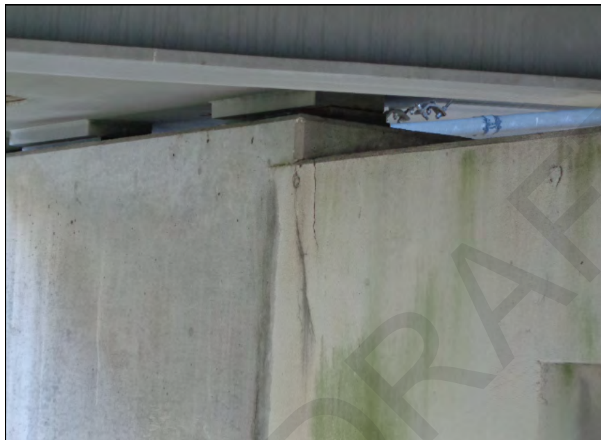
PHOTO 21 – ELEMENT 234 VIEW OF 16 IN. VERTICAL CRACK, SOUTH FACE OF PIER CAP 1, ADJACENT TO PEOPLE MOVER EXTENSION
