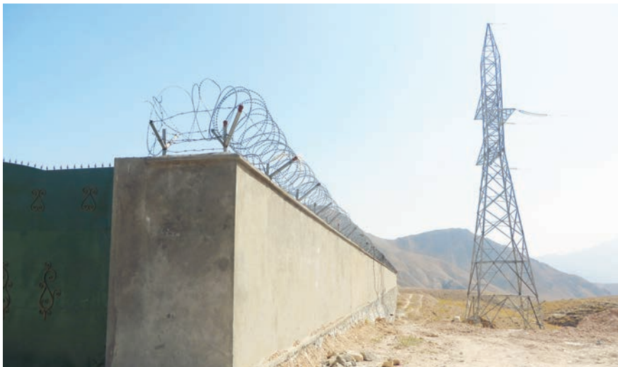
A Northeast Power System terminal tower ending without connection to the Nejrab District substation. (SIGAR photo)
