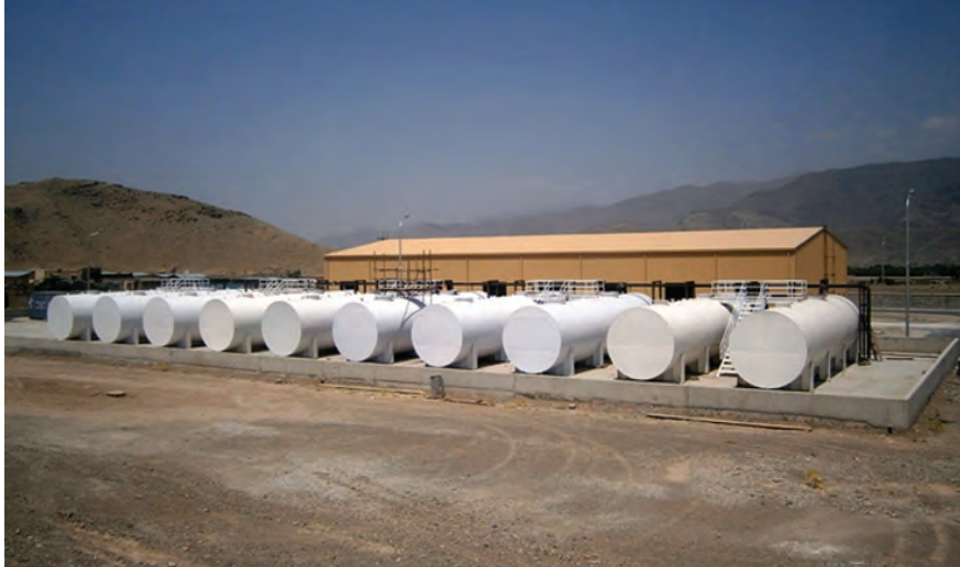
An ANA 201st Corps electrical power-plant fuel farm was built in Kunar Province. (CSTC-A photo)
