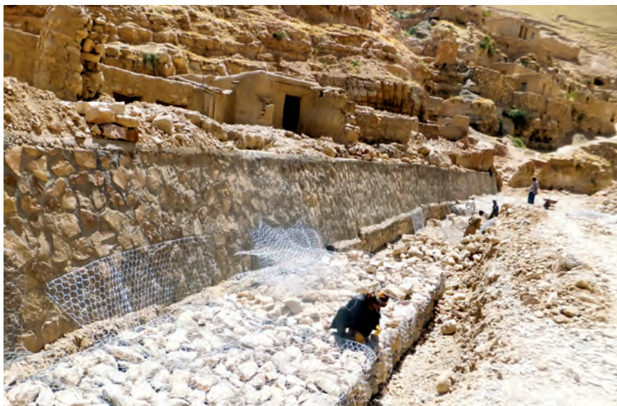
A SIKA West-sponsored flood-protection wall being constructed by the community in Badghis Province. (USAID photo)
