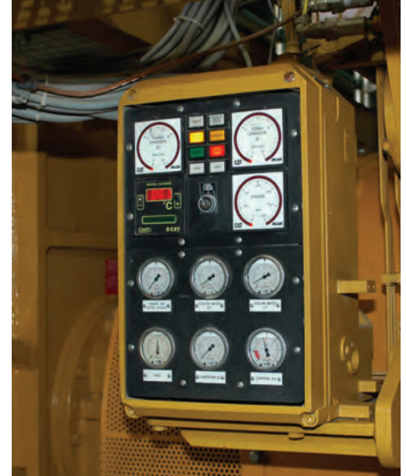
SIGAR's Office of Special Projects continues to review the use of the $335 million Tarakhil Power Plant. Seen here, a control panel at the plant. (USAID photo)
