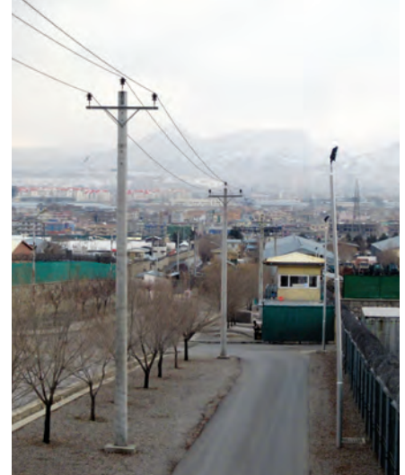
A SIGAR inspection of a power-grid project, including these overhead power lines, at the Counter Narcotics Strip Mall found that although the State Department accepted the project from the contractor, the electrical system powering the compounds was not tested and deemed operable until more than 18 months later. (SIGAR photo)
