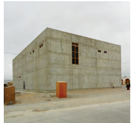
A SIGAR inspection found that while the exterior of the command-and-control facility at Camp Brown was solidly built and without cracks, the interior was a shell with no flooring, electrical, or plumbing systems, or any means of ascending to the second floor. (SIGAR photo)
