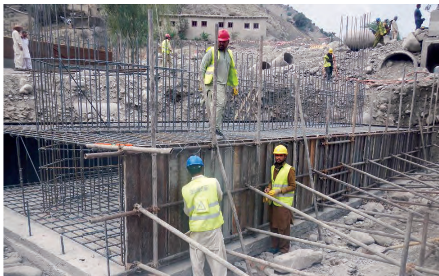
Workers construct the footing for a bridge that is part of the Gardez-Khowst road rehabilitation project. (USAID photo)
