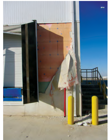
SIGAR's inspection of a warehouse at KAF found several minor construction deficiencies, including exterior siding torn away from the building. (SIGAR photo by Ronald Snyder)
