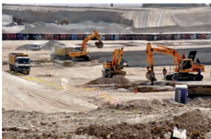
At a U.S. Army Corps of Engineers project, heavy equipment prepares ground for a facility to house Afghan soldiers. (U.S. Army photo by Mike Beeman)
