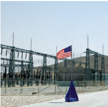
USAID invested $355 million on the Tarakhil Power Plant, which is the subject of a SIGAR inquiry letter this quarter. (USAID photo)
