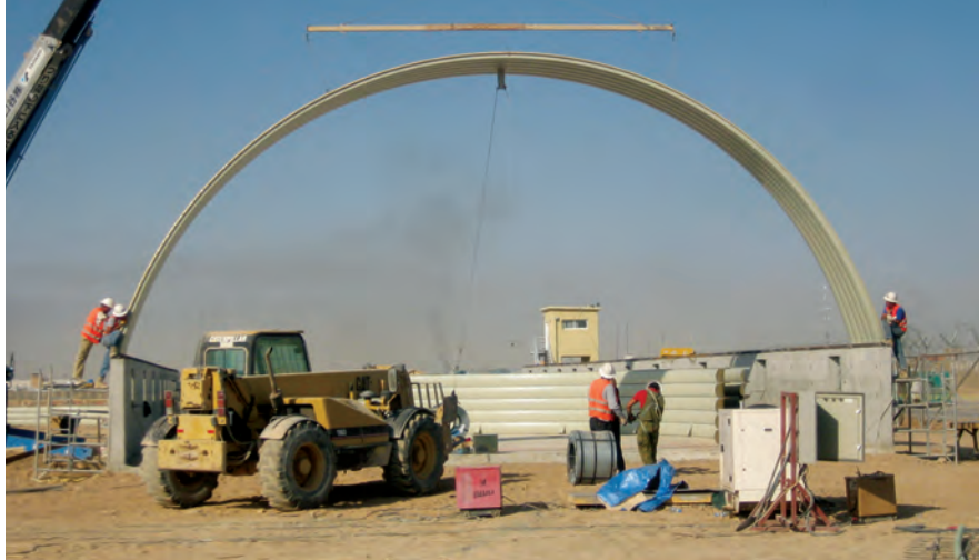
Building assembly begins at a facility for the Afghan National Army. (U.S. Air Force photo)
