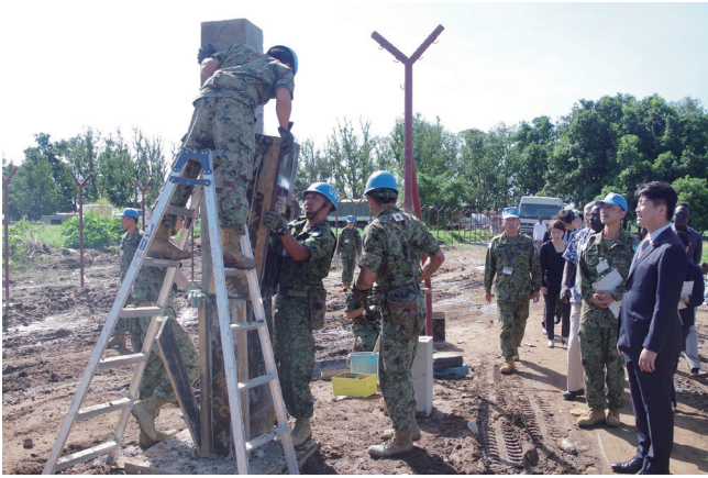
Parliamentary Vice-Minister Ishikawa inspecting the Juba River Port Security Fence construction work in South Sudan
