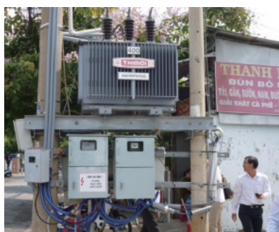
Photo 1 Introduction of high efficiency transformers in power distribution systems in Vietnam
