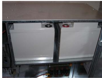
Figure 3 - 24 Vdc monoblocs series installation
