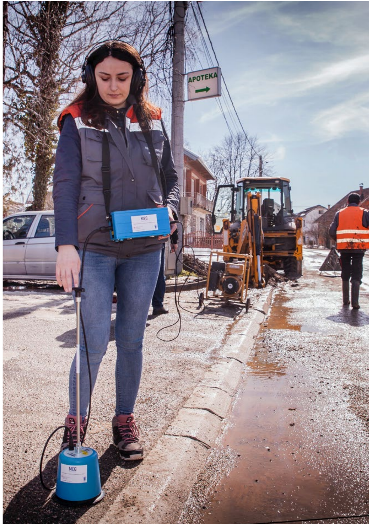
Repairing water pipes: Authorities are supported to provide better access to drinking water and ensure waste water treatment. Municipal Governance and Environment Project, Kostajonica.
