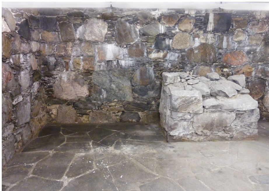
Fig. 7.12: The royal palatium at Holmen. The residential quarter from the late 13th century, facing Vågen. Northern part of the eastern wall, view from west. The lower part is original, the upper part restored, and the transition is visible as small green spots (brass pins). The pillar is secondary. Photo: A. T. Hommedal.
