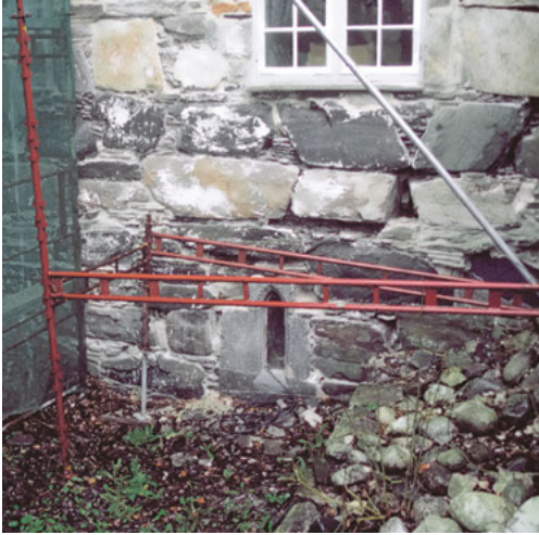
Fig. 7.24: One of the two original pointed windows to the cellar. Photo: A. T. Hommedal.
