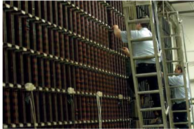
Fault management by OTE technicians
