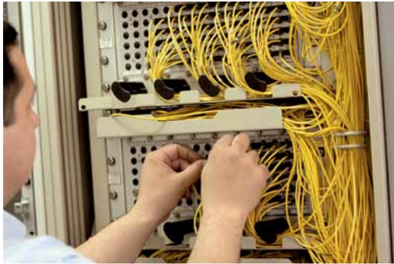
Fault management by OTE technicians
