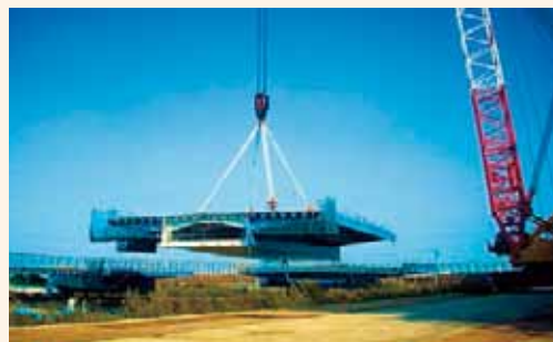
A Taiyo Seiki heavy round sling being put to use at a bridge-building site
