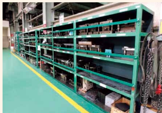
A metal storage area outfitted with apparatus to prevent items from falling
