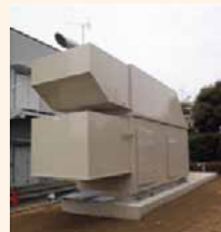
Power generator installed after the 2011 earthquake
