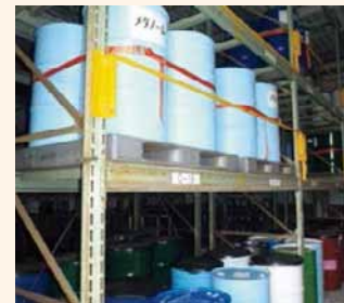
The seismic mitigation racks installed on March 7, 2011, that prevented damage in the earthquake that followed
