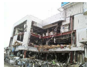
Damage state of Takada branch
