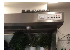
Electrical equipment placed in upper area
