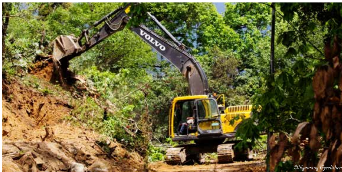
Road construction in Gasa, 2014. Land allotted for construction of power transmission lines and roads accounted to 49 per cent of the GRF land allotted for development activities from 2008-2013
