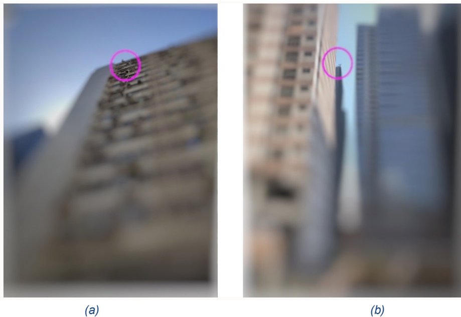
Figure 4 What appeared to be 5G base stations installed (a) on the rooftop of the same building above the TVRO antenna and (b) on the rooftop of an adjacent building in the pointing direction of the TVRO antenna.
