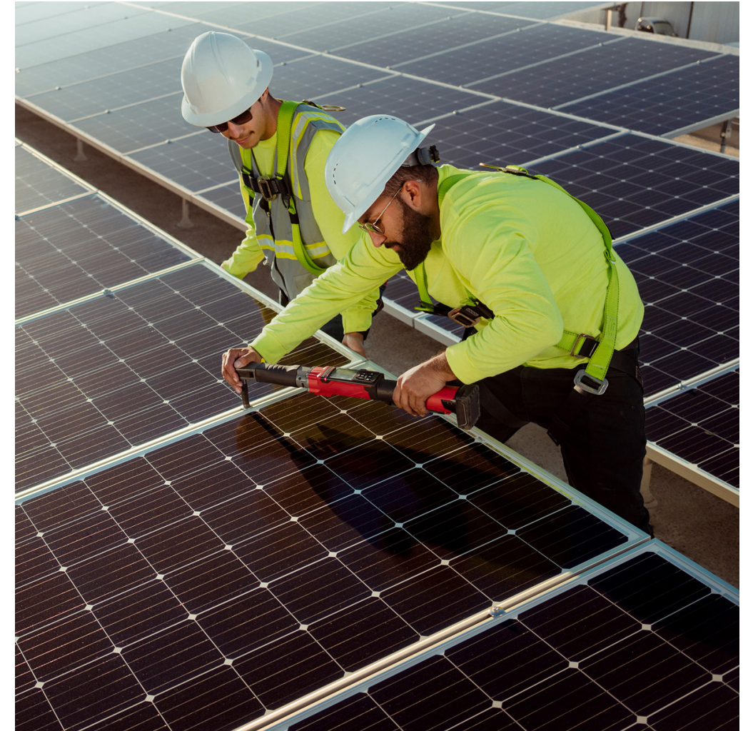
Technicians from Simmitri perform maintenance on solar panels installed at Bench-Tek Solutions in Santa Clara, California. Both companies are alumni of the Apple Impact Accelerator.
