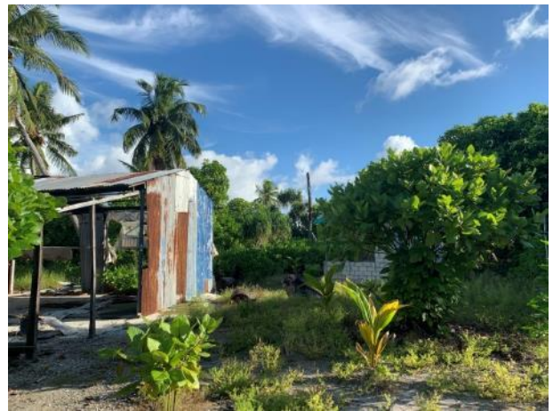
Figure 35.4: The buildings found at the site have been vandalized over the years and are not in a usable state
