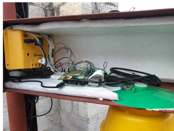
Fig. 11: Housing case for the Charge Controller, Raspberry PI 3 Model B+ and Arduino Uno Rev 3
