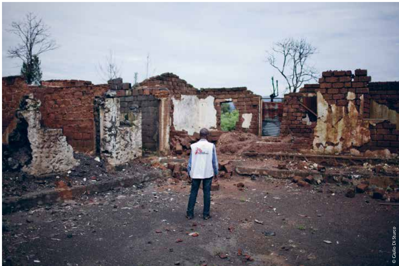
A staff member surveys what remains of the MSF office in Kitchanga, Democratic Republic of Congo, after a wave of violence engulfed the town.
