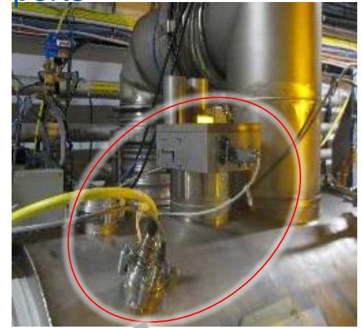
Vac instrumentation ports
