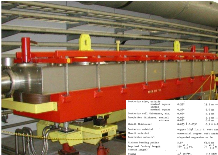
MSSB splitter magnet (CERN) MgO MIC water-cooled cable
