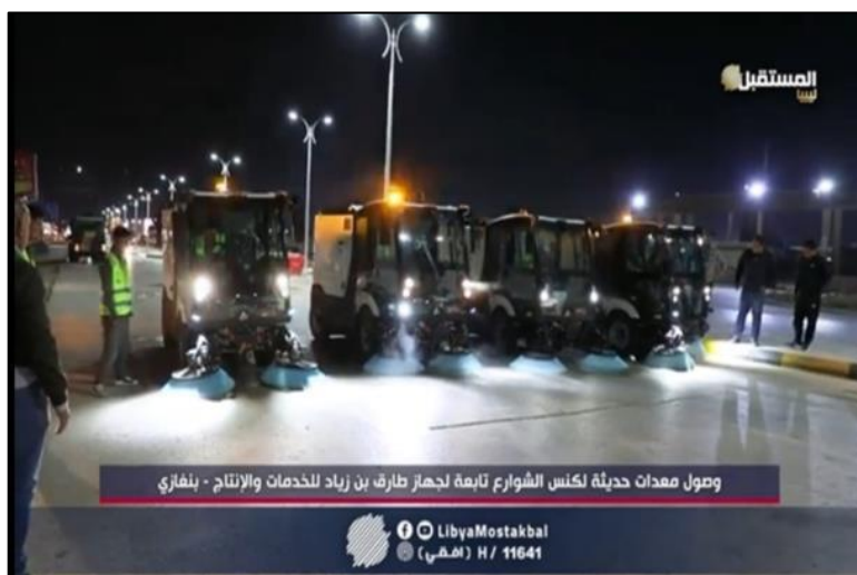
Figure 12.1 Road Maintenance in Benghazi
