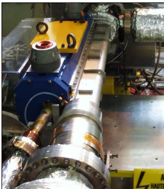
Figure 2: LEIR extraction magnet (blue) installed in the ring.
